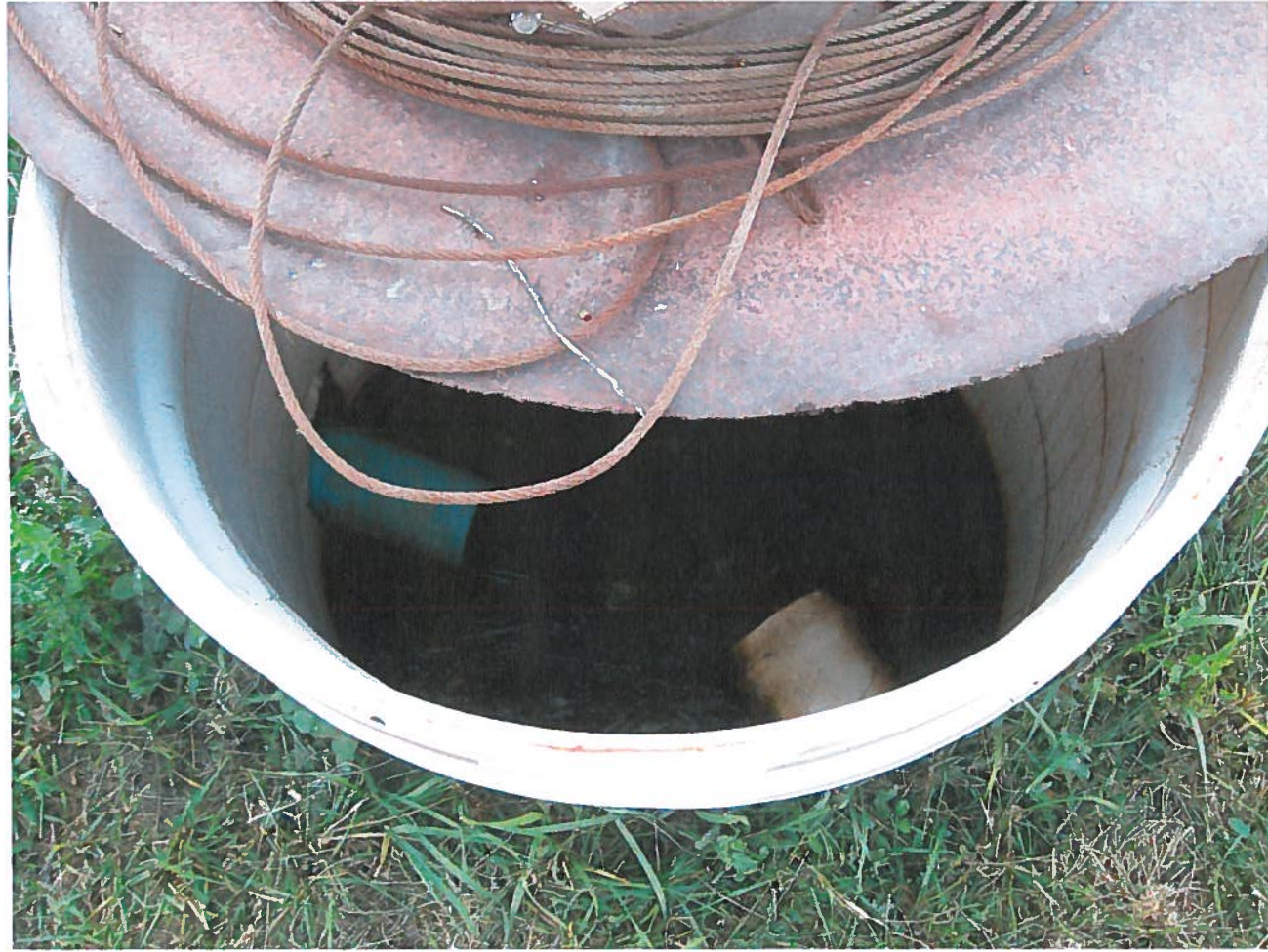
Transfer box on tile drain system.
