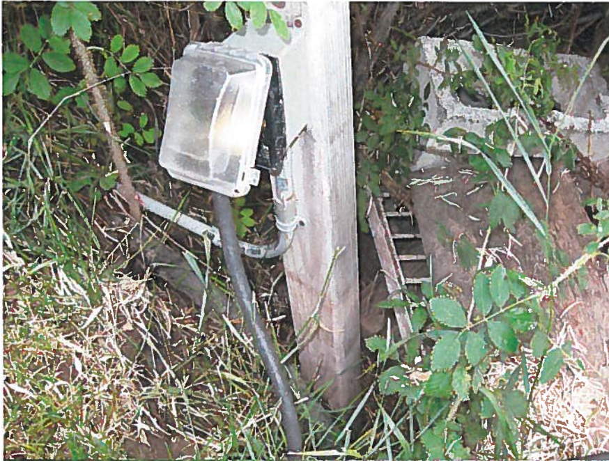
Power to the pump
