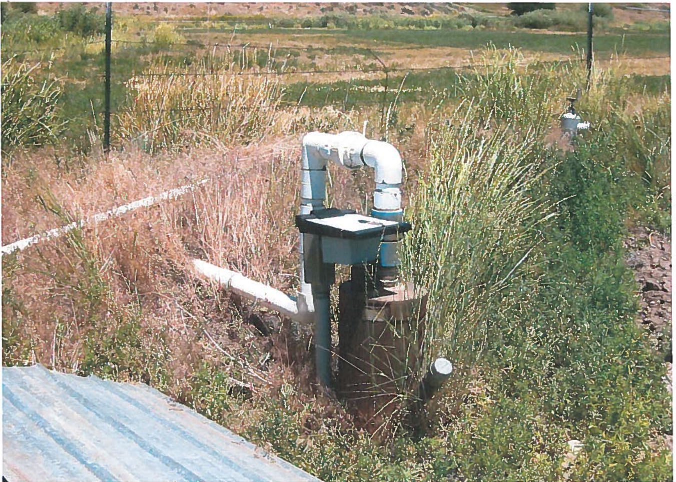
well with irrigation pipe
