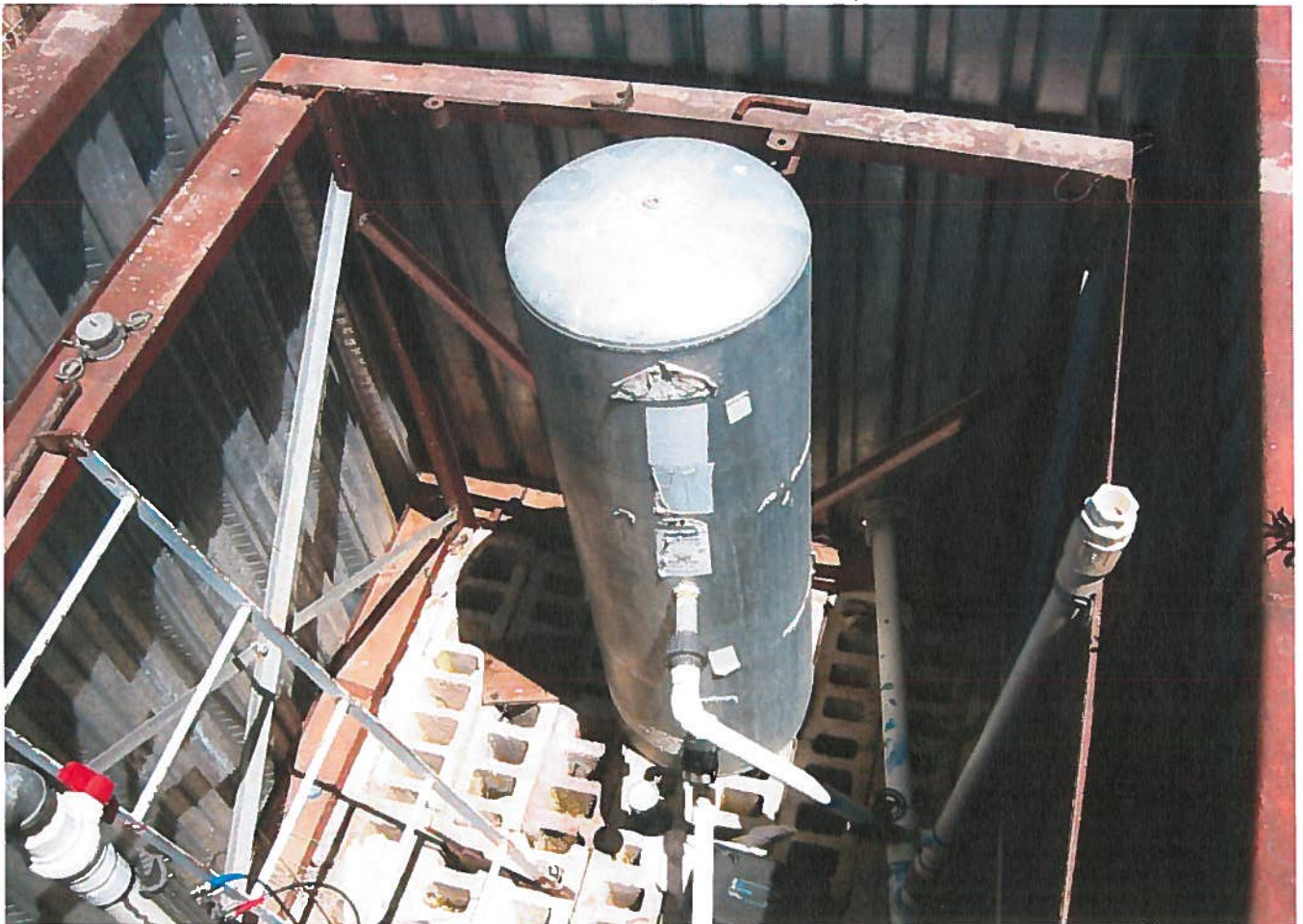
Pump house (Underground) and fish pond plumbing
