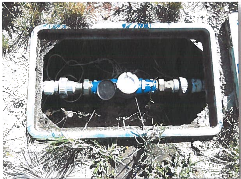
Figure 5 Picture of DLJ Flow Meter
