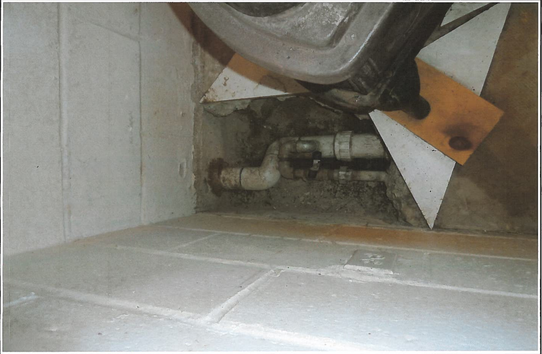
FIGURE 6: SUPPLY LINE ENTERING THE HOUSE AND VALVE FOR HEATING RUSSELL THOMPSON PERMIT NOS. 47-7578 AND 47-7579
