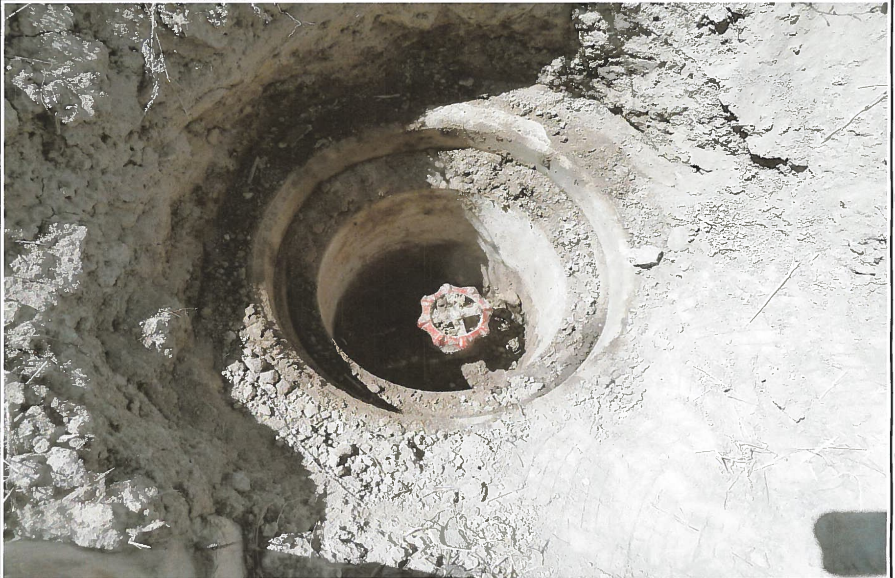
FIGURE 7: VALVE TO IRRIGATION AND RECREATIONAL POND RUSSELL THOMPSON PERMIT NOS. 47-7578 AND 47-7579
