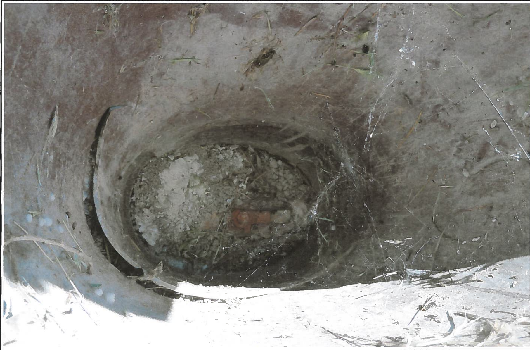
FIGURE 8: IRRIGATION SYSTEM VALVE RUSSELL THOMPSON PERMIT NOS. 47-7578 AND 47-7579 SITE VISIT ON 6/8/2012
