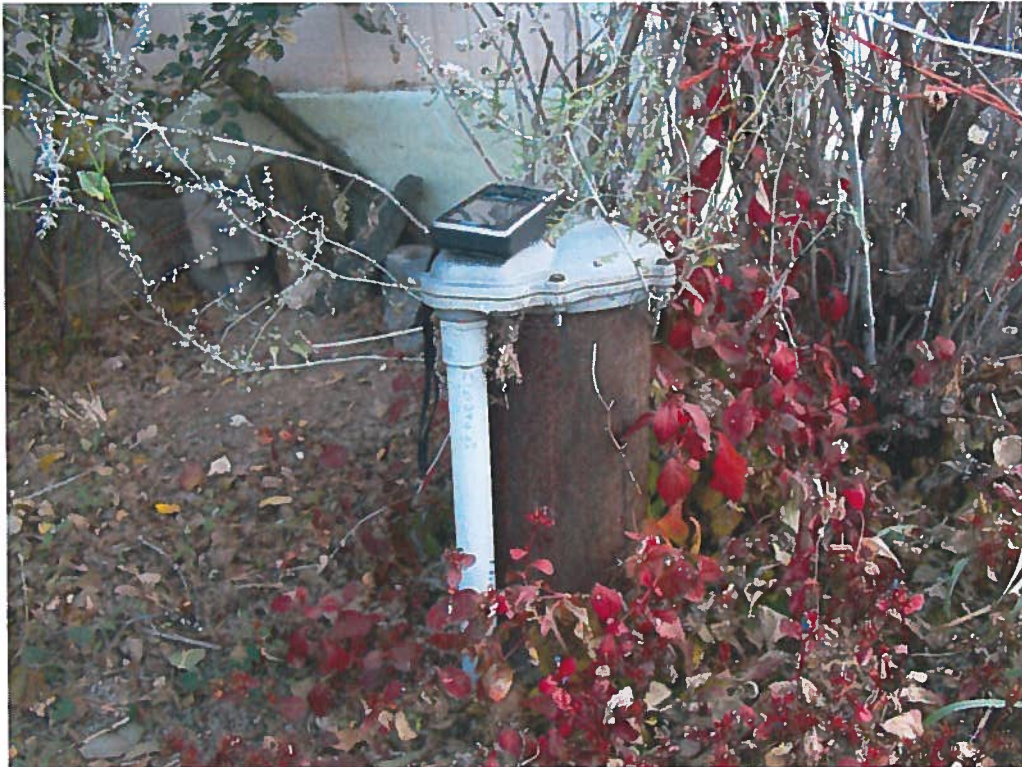
63-12115 Exam 11/8/2012: P/D well with pump house/shed in background facing southwest.
