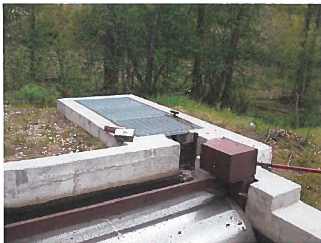
This photo shows the fish screed with the orifice handle sticking up through the grate at the top of the photo.
