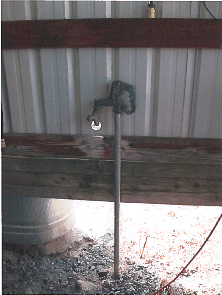
Hydrant in the barn.
