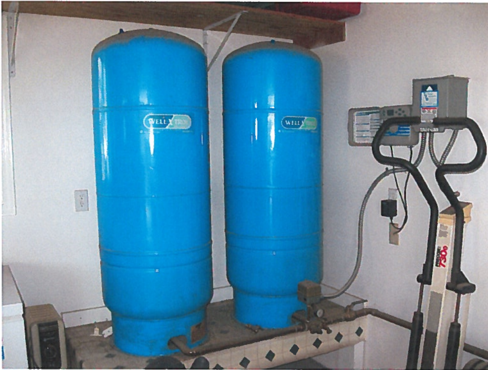
Inside garage, 2 pressure tanks and automatic sprinkler controls.
