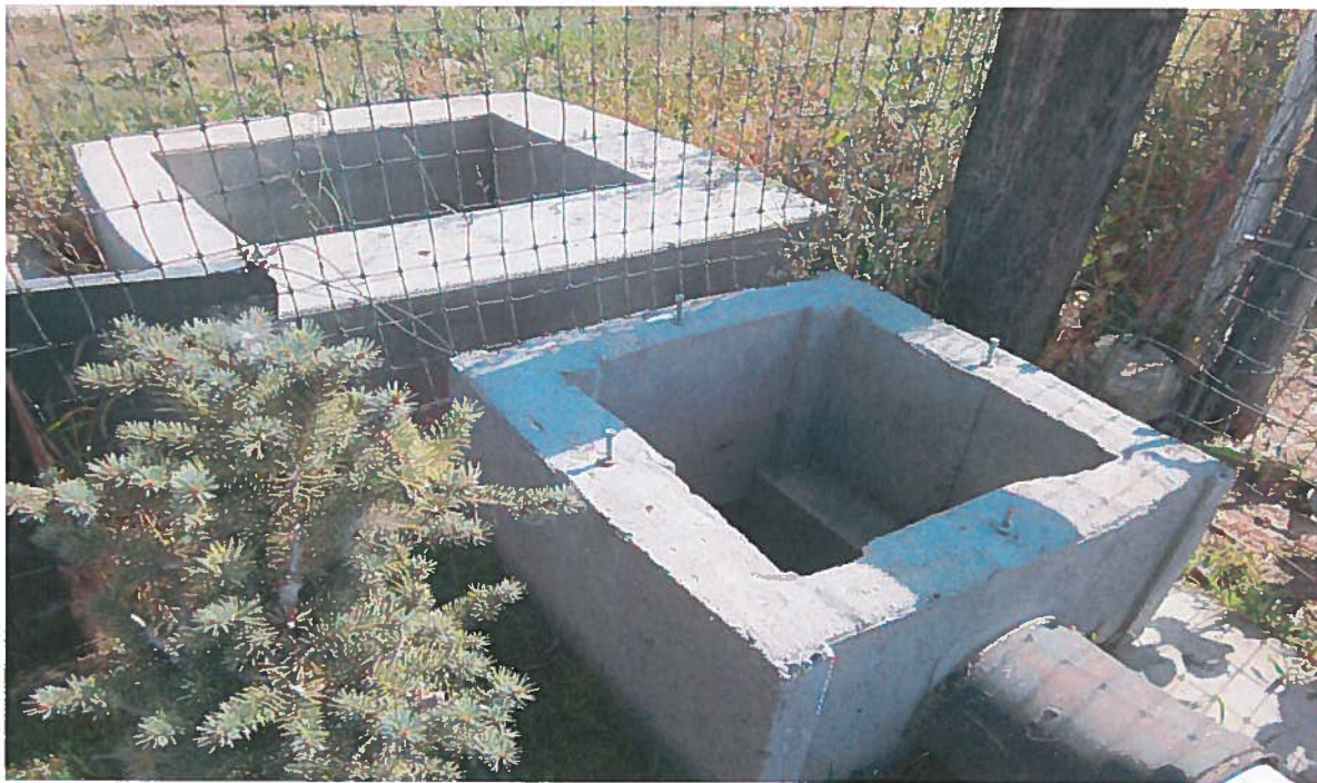
Concrete vault and headgate across fence is on the ditch. Water piped to water users headgate and to the gated pipe to flood irrigate the field.
