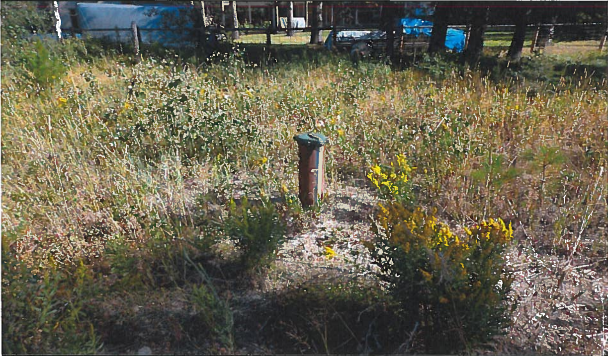
Point of Diversion (New Well): View northerly of domestic and irrigation ground water well.
