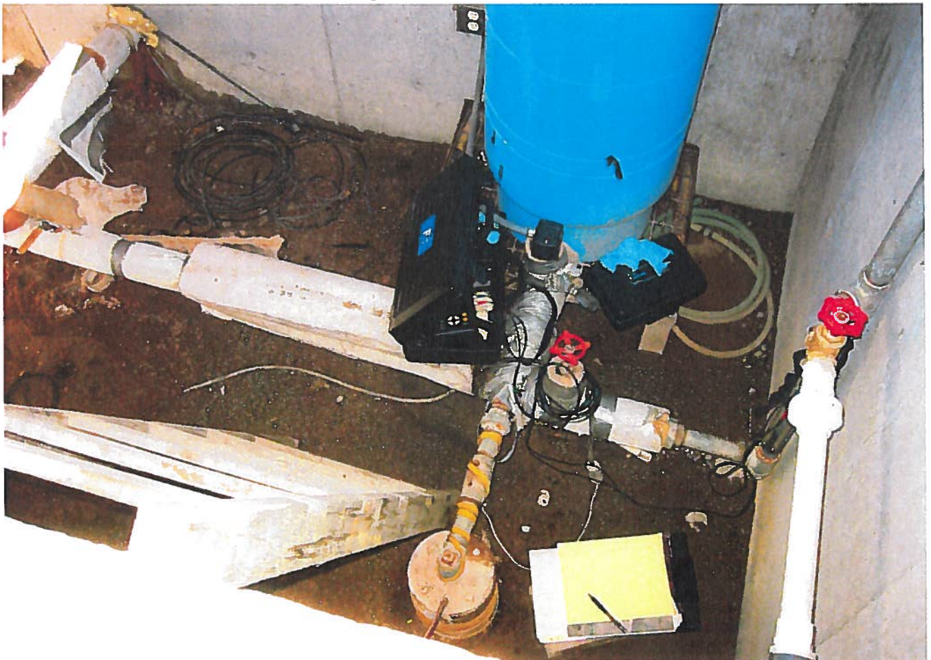
Inside well house- 11-7212
