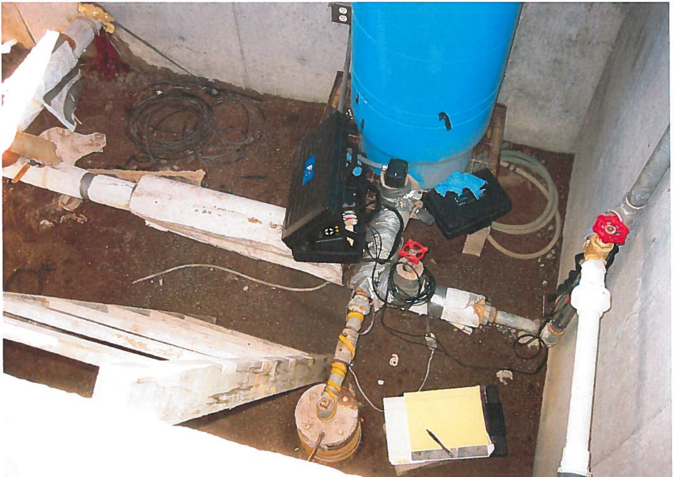
Inside well house - 11-7212
