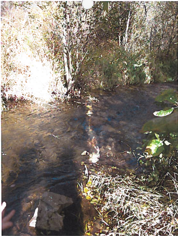
A smaller pipe is encased in the pipe shown in this photo
