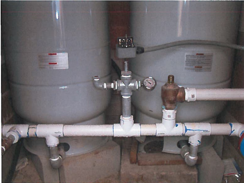
63-31597 Exam 9/6/2012: Pressure tanks in-line between flow meter and discharge lines to buildings inside pump house.
