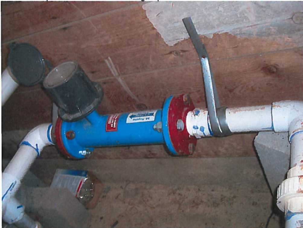
63-31597 Exam 9/6/2012: Flow meter in-line between intake from well into pump house and pressure tanks.
