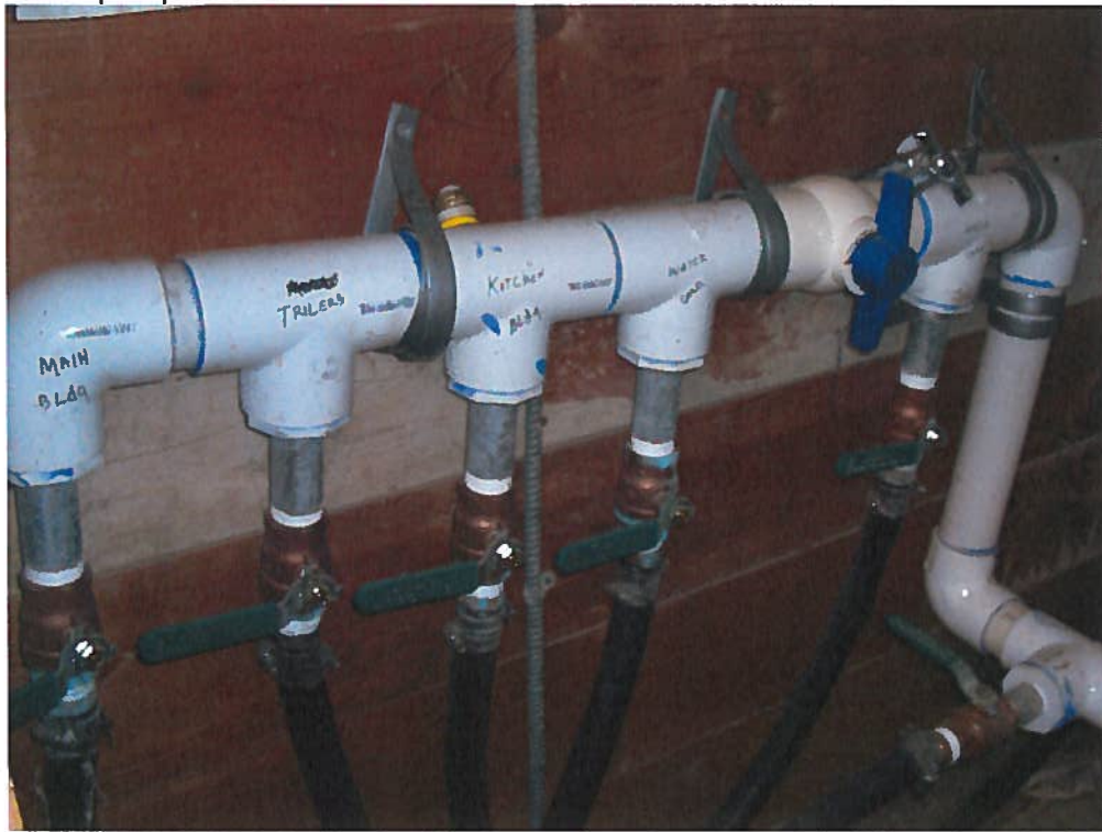
63-31597 Exam 9/6/2012: Distribution/discharge lines into school buildings from inside pump house.
