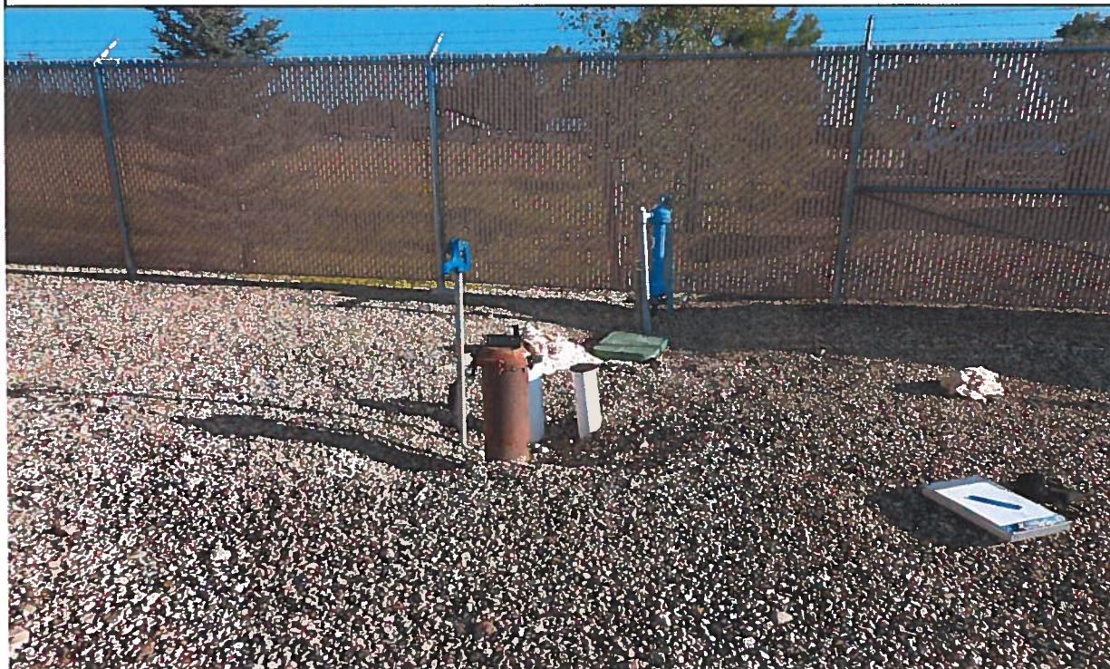
Point of Diversion: View northwesterly of irrigation ground water well. Pump house is located 10 – 15' west of well.
