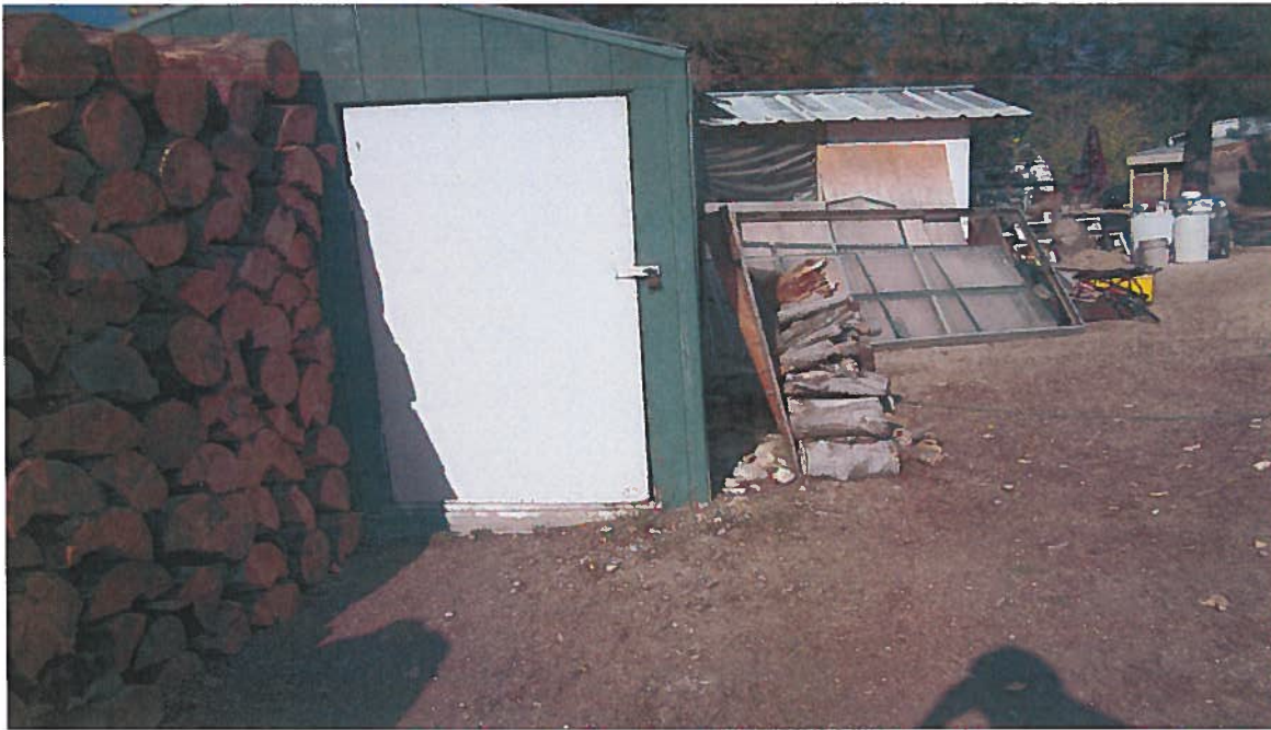
The pump house behind the Longpre main house.
