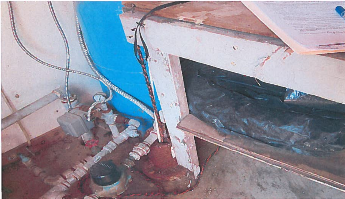
The well and associated piping. One of the blue pressure tanks seen.
