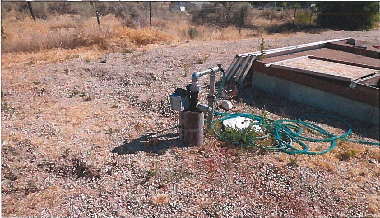
Point of Diversion: View northeasterly of ground water well. Well contains two submersible pumps – A 2hp for domestic use for one home, and a 5hp pump for irrigation. A subsurface pump house/vault is shown easterly of well.
