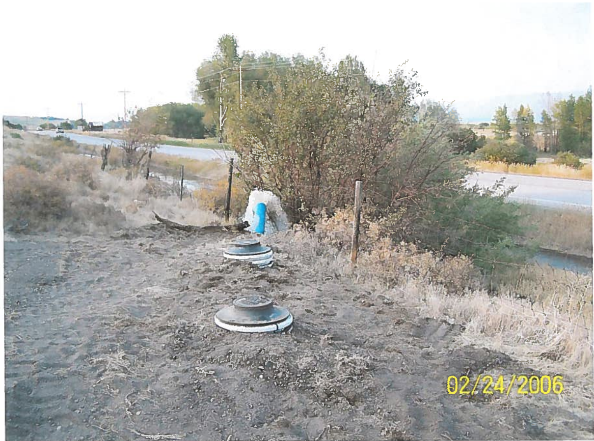
Terminus of the Sam's Hollow mitigation pipeline.
