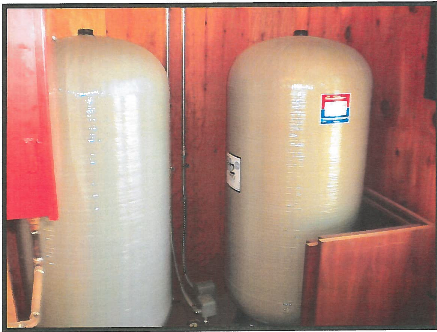
Domestic system pressure tanks
