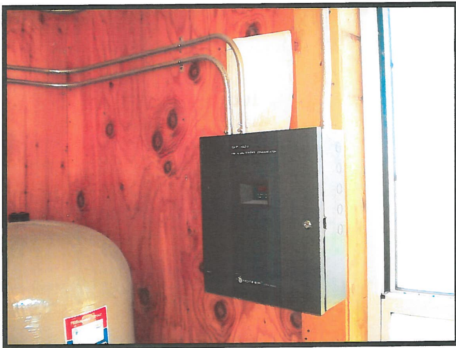
Fire alarm control monitor
