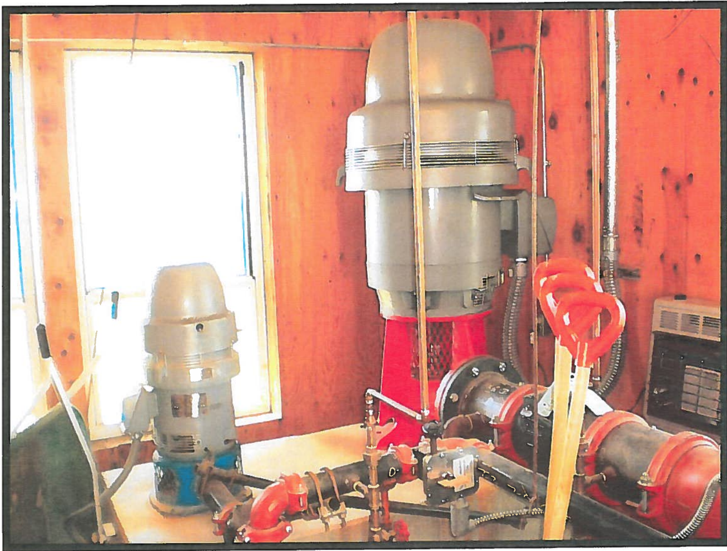
Fire system booster pumps
