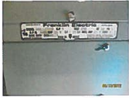
PUMP IN WELL.JPG
