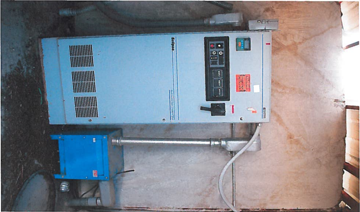
Inside pump house
