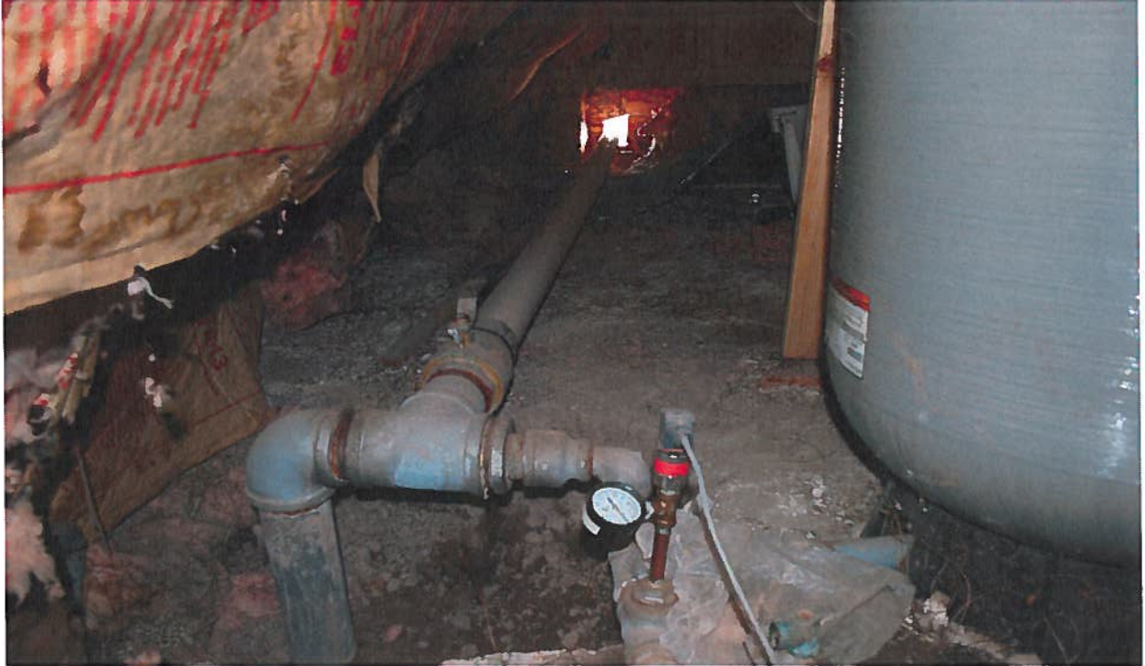
Inside of Pump House
