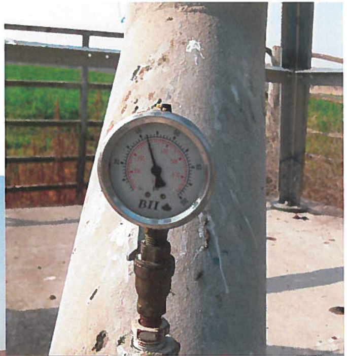
45psi is the pressure reading at the large pivot
