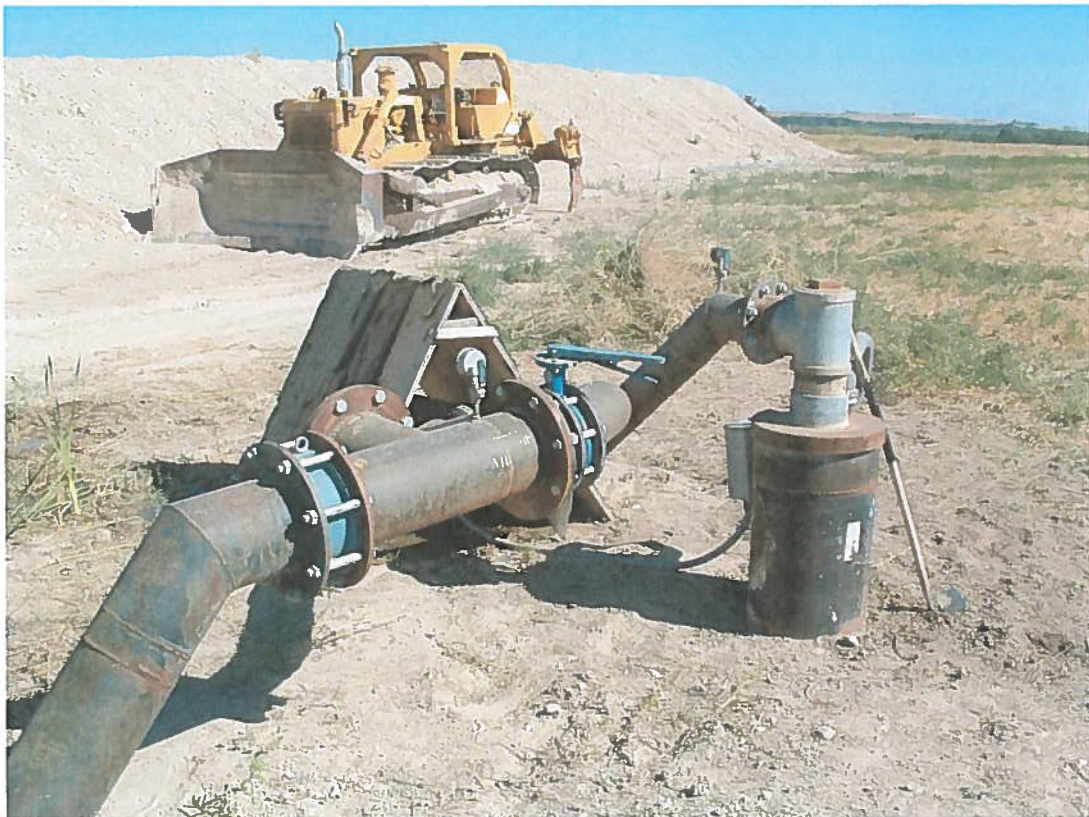
Well 1; 20-hp booster pump beneath A-frame sun shade.
