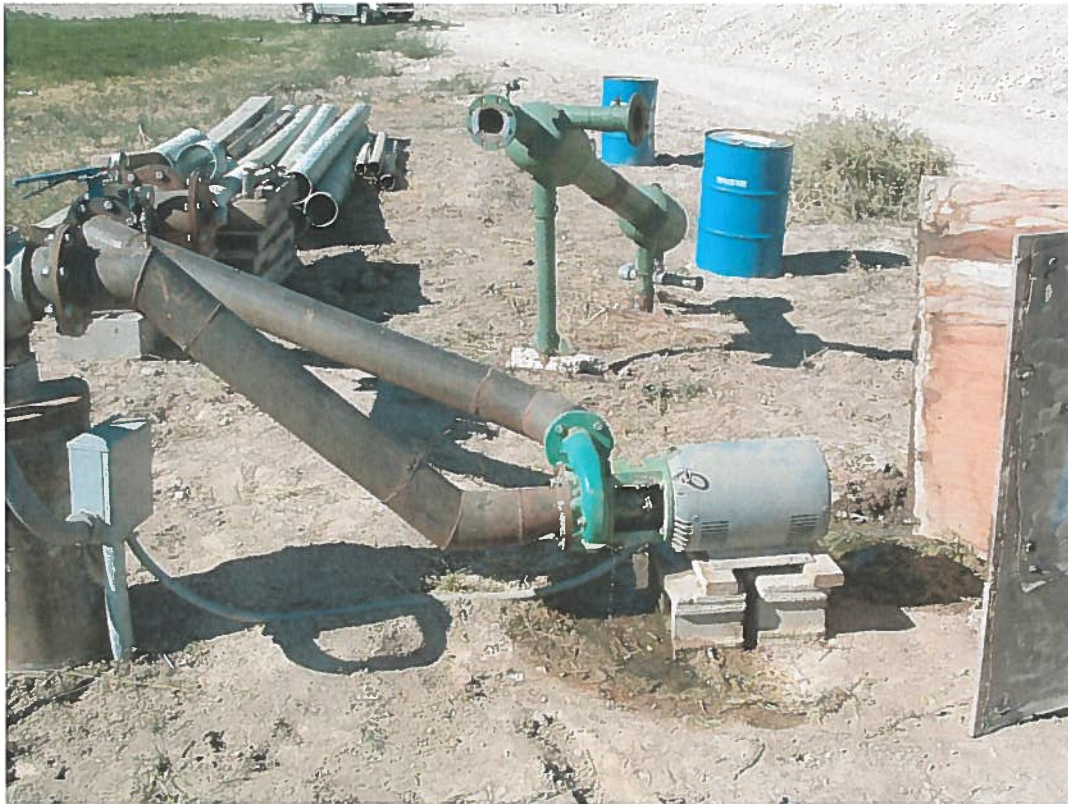
Well 1 20-hp booster pump (with sun shade removed)
