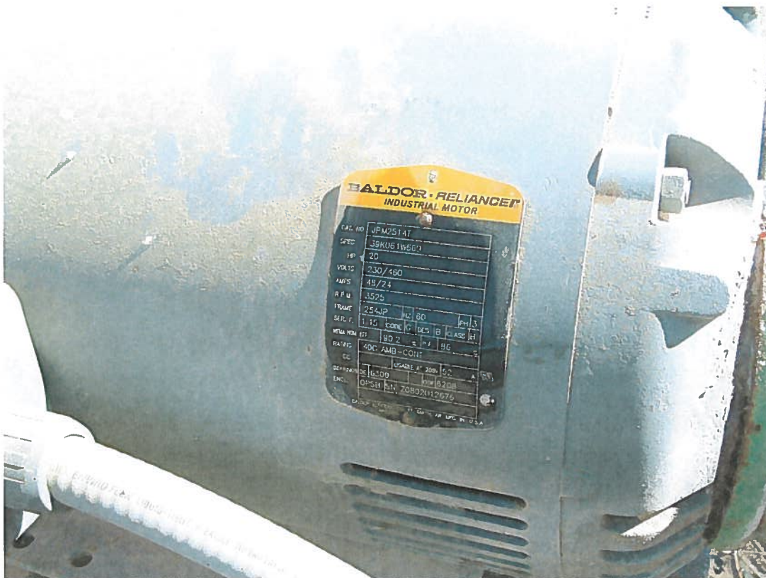
Well 1 booster pump motor nameplate
