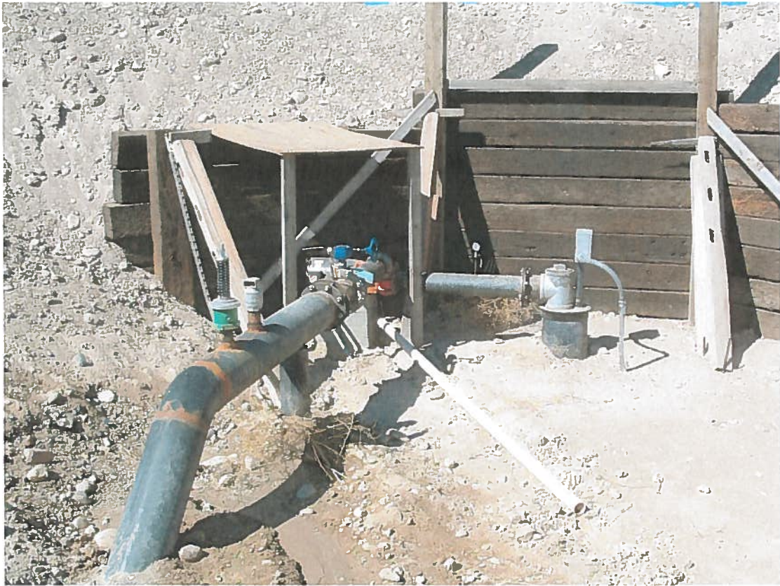
Well 2 discharge piping
