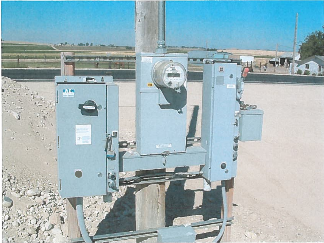
Well 1 Motor Controls
