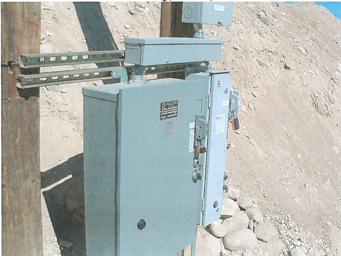
Well 2 motor controls
