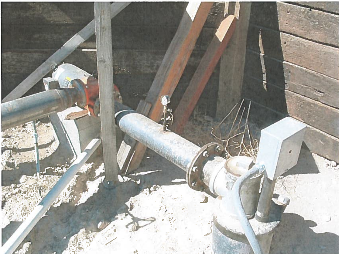
Well 2 (lower right) and 15-hp booster (upper left)
