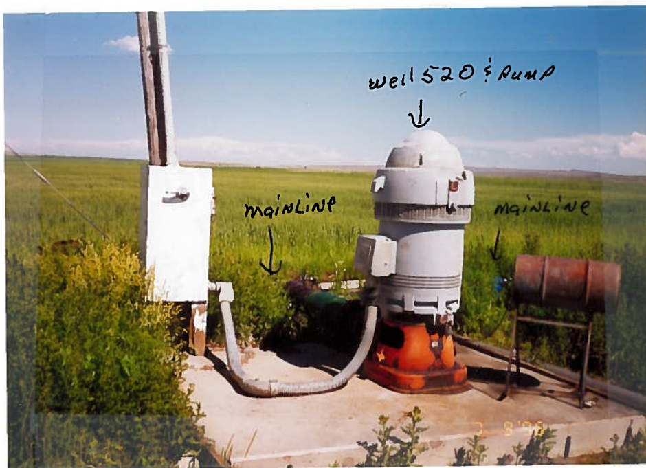
Well # 520. Pump Diverts water into a North and South mainline. The mainline has a spur on it that goes to the west
