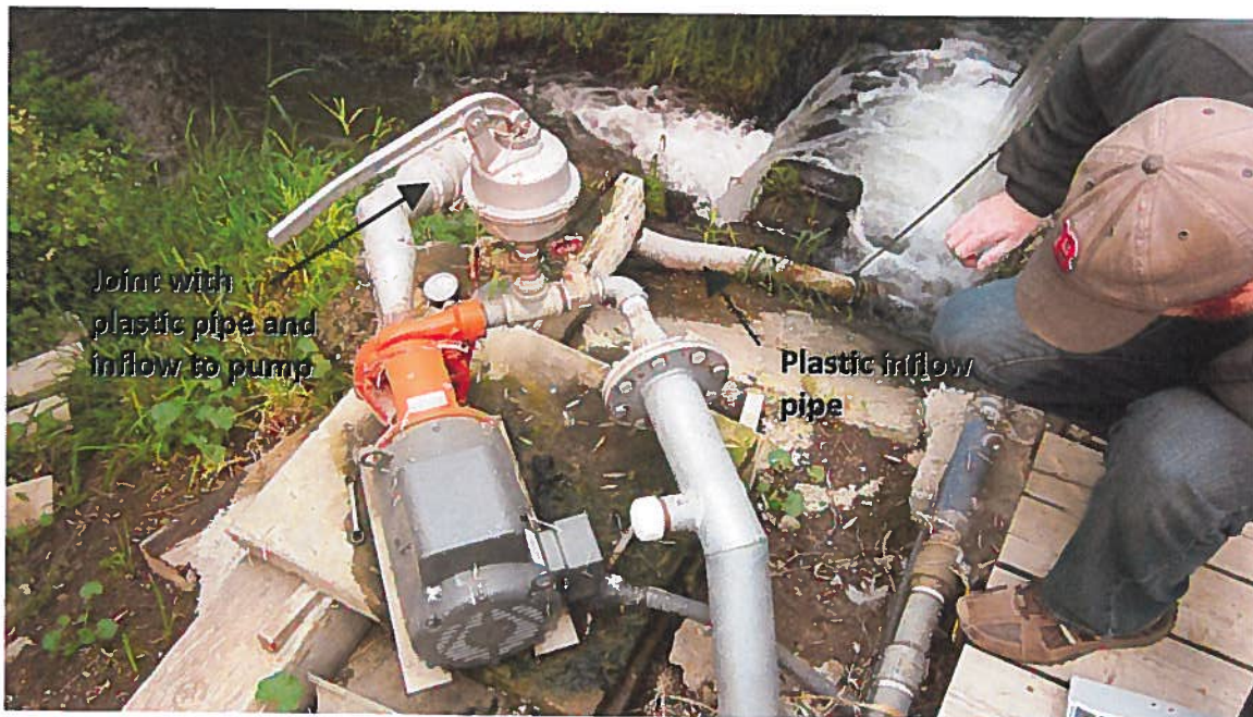
Licensed POD – Looking at the pump and corrugated plastic pipe pulling water from the unnamed drain.
