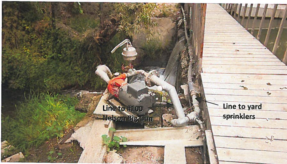
Licensed POD – Looking north across the unnamed drain showing the 7.5 HP Baldor Reliance pump and discharge pipes.
