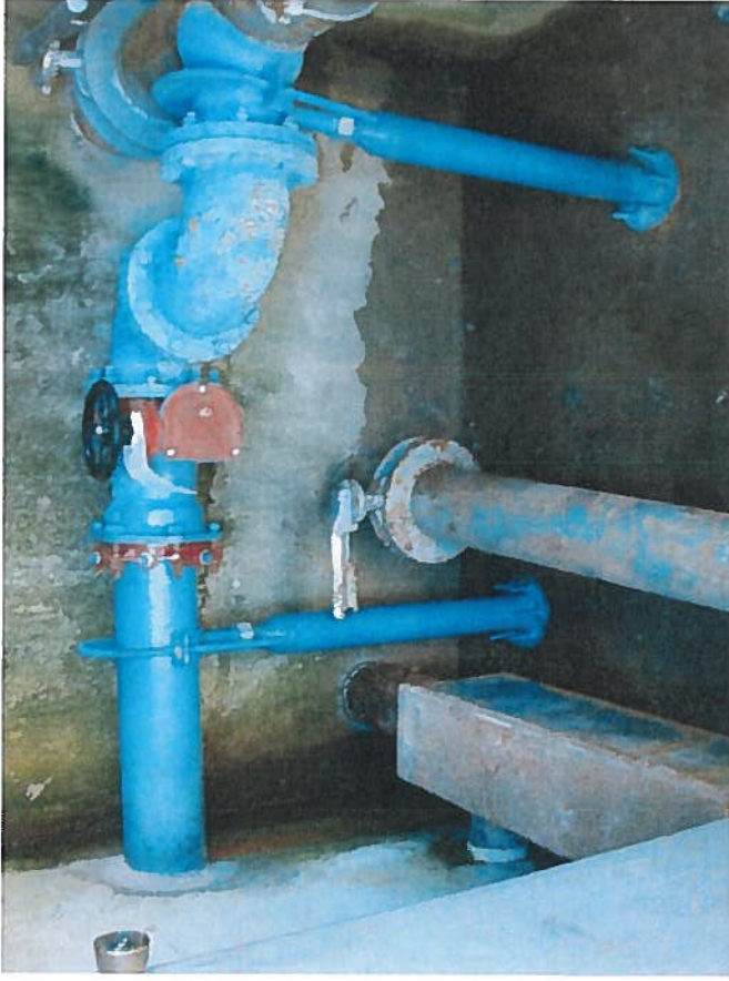
24. Inlet from Tank 2 (R), tank 1 back (L), overflows & drains below
