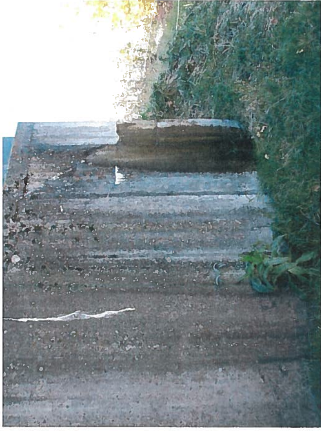
Photo #2. Tank #1 Leaking at the North West corner
