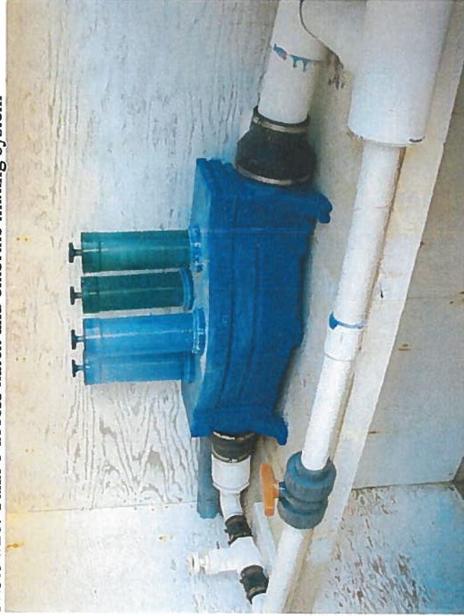
Photo #30. Chlorine pellet erosion contact chamber
