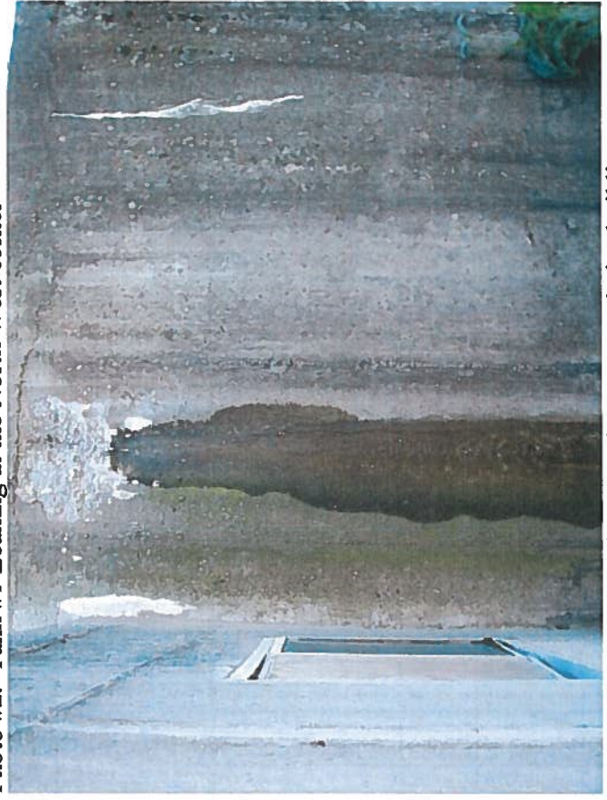
Photo #4 Tank #1 leaking near the connected pipe building
