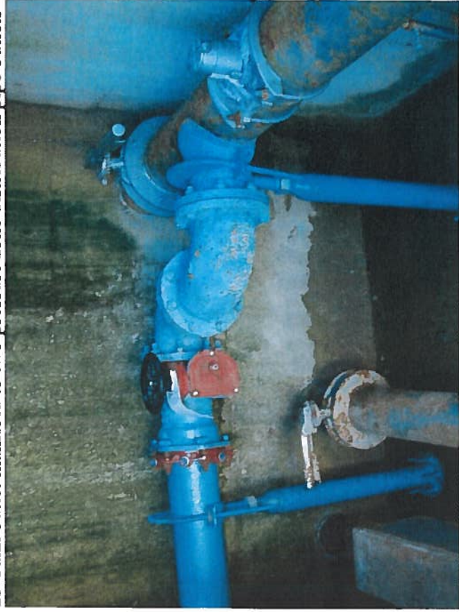
Photo #27. Isolation valves for each tank
