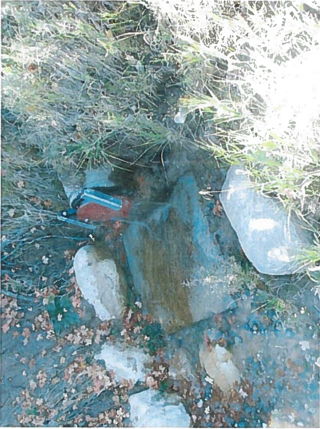
Photo #32. Combined tank overflow over the splash plate
