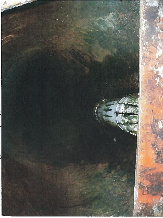
Photo #41. View of overflow up the pipe
