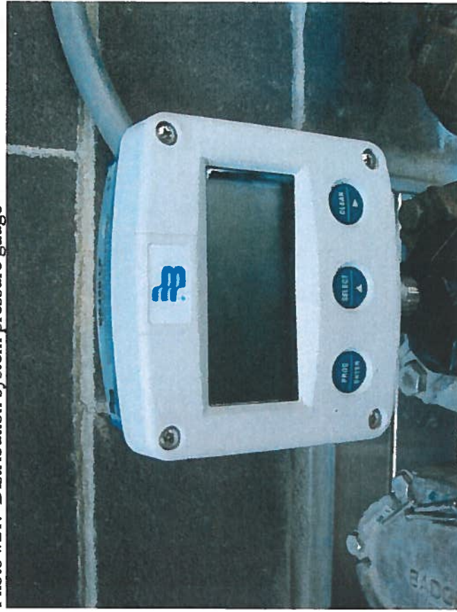
Photo #23. Flow meter digital readout
