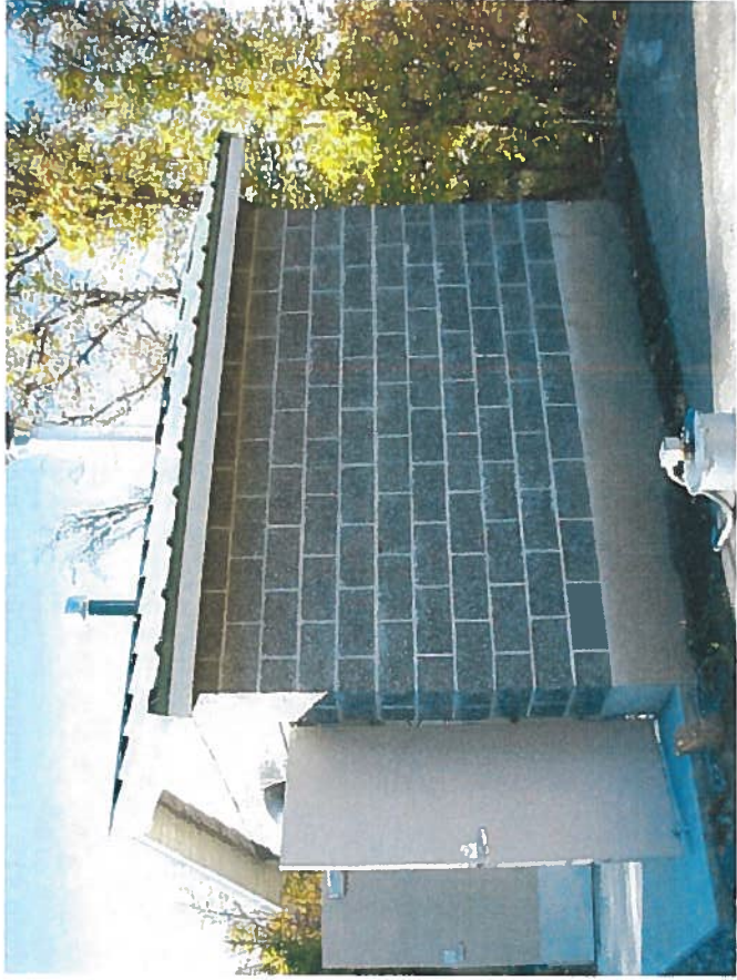
Photo #13. New Chlorine Building facing south, also tank level sensor
