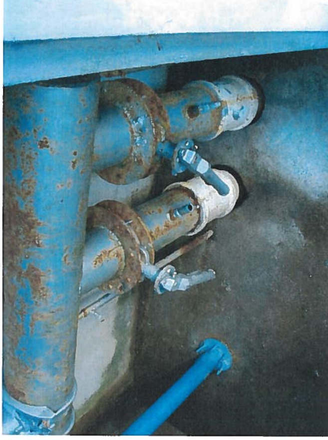
25 Tank outlet manifold to two pressure zone distribution pipe outlets
