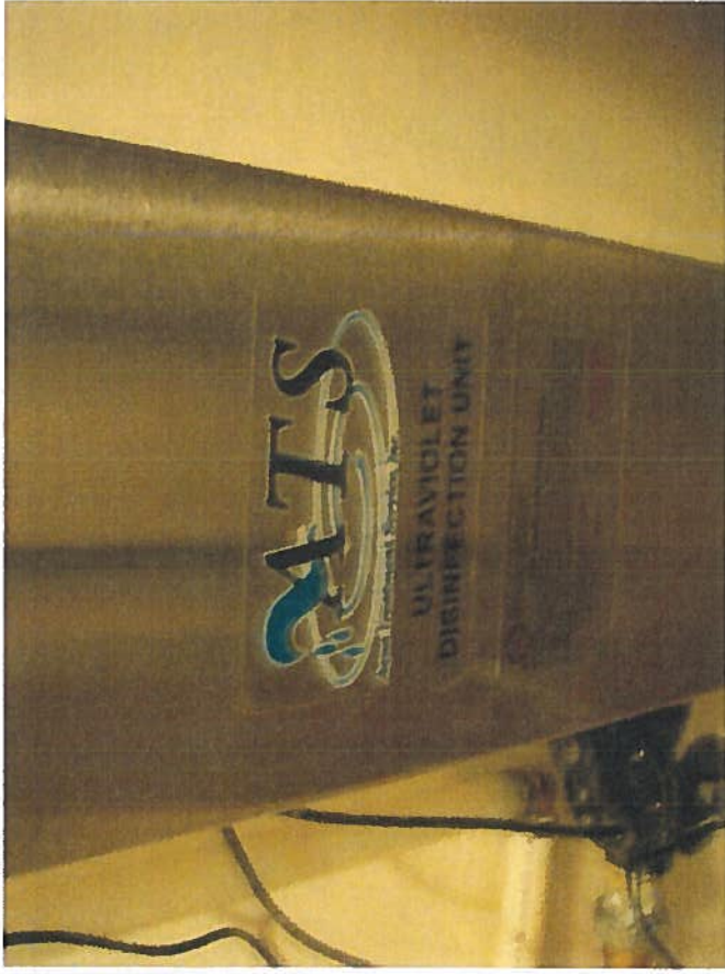
Photo #35. UV disinfection unit – private residence
