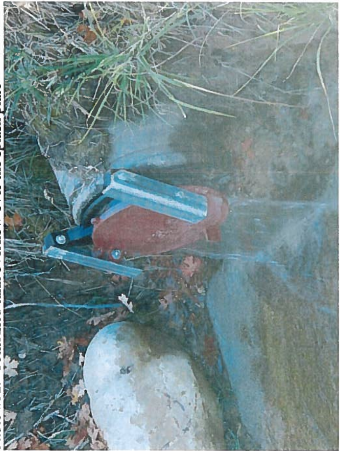
Photo #34. Close up of water overflow, un-chlorinated
