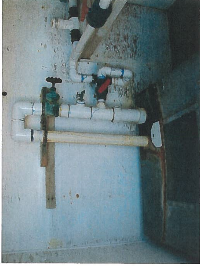
Photo #29. Current chlorine supply for chlorinator
