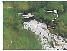
STAND UP PIPE AT CANNEL.jpg
