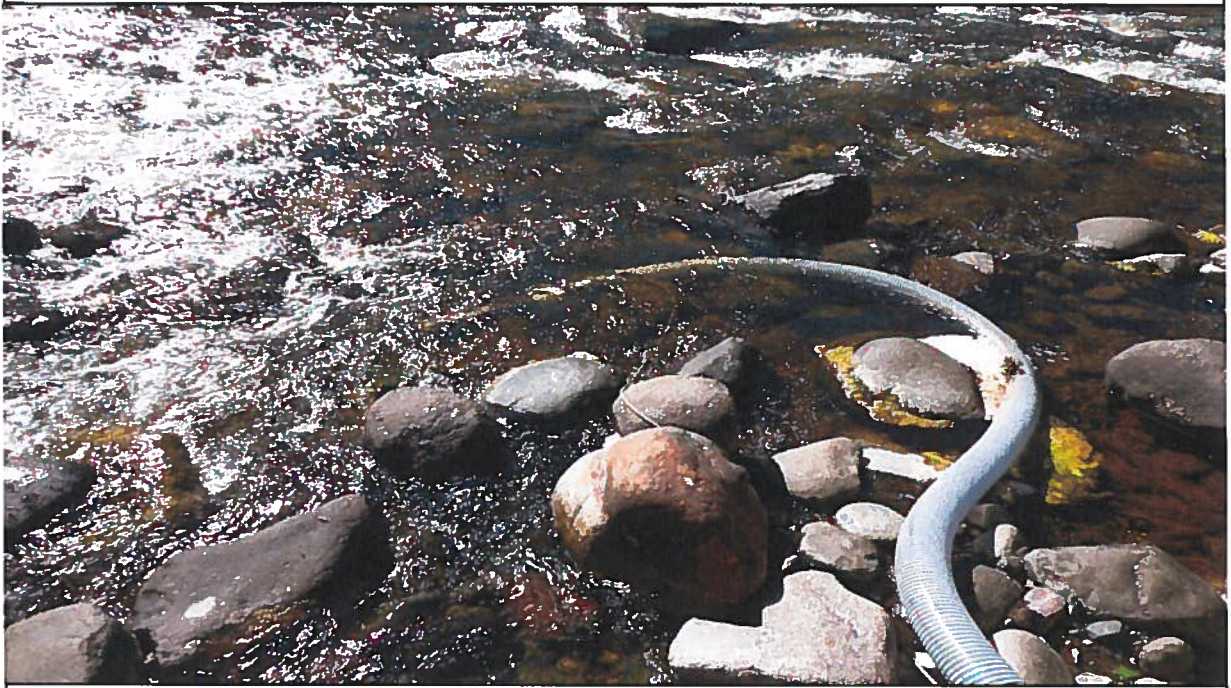
Point of Diversion: View westerly of screened 4" Flexible Pipe suction line in the Little Salmon River. The suction line connects to a 4" PVC line to the pump house.
