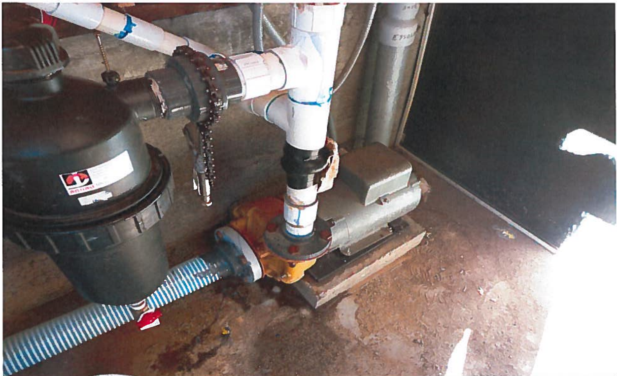
View inside of pump house of 10 hp pump and motor and 4" suction line from the Little Salmon River.
