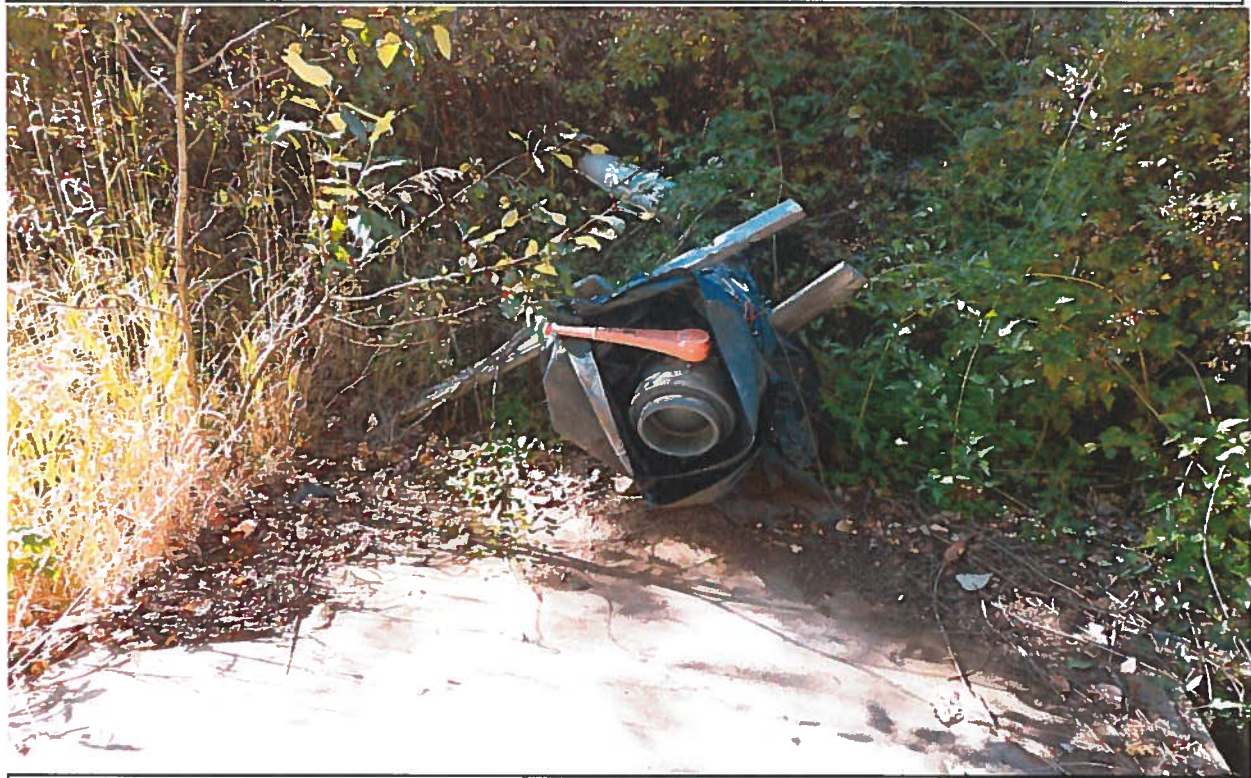
View southwesterly of the terminus of the 6" PVC conveyance pipe. The 6" valve remains closed during the irrigation season to maintain pressure head in the pipe for irrigation. At the end of the irrigation season, the 6" valve is opened to drain the pipe onto the concrete slab. The water sheets off the concrete slab and discharges back to Fall Creek.
