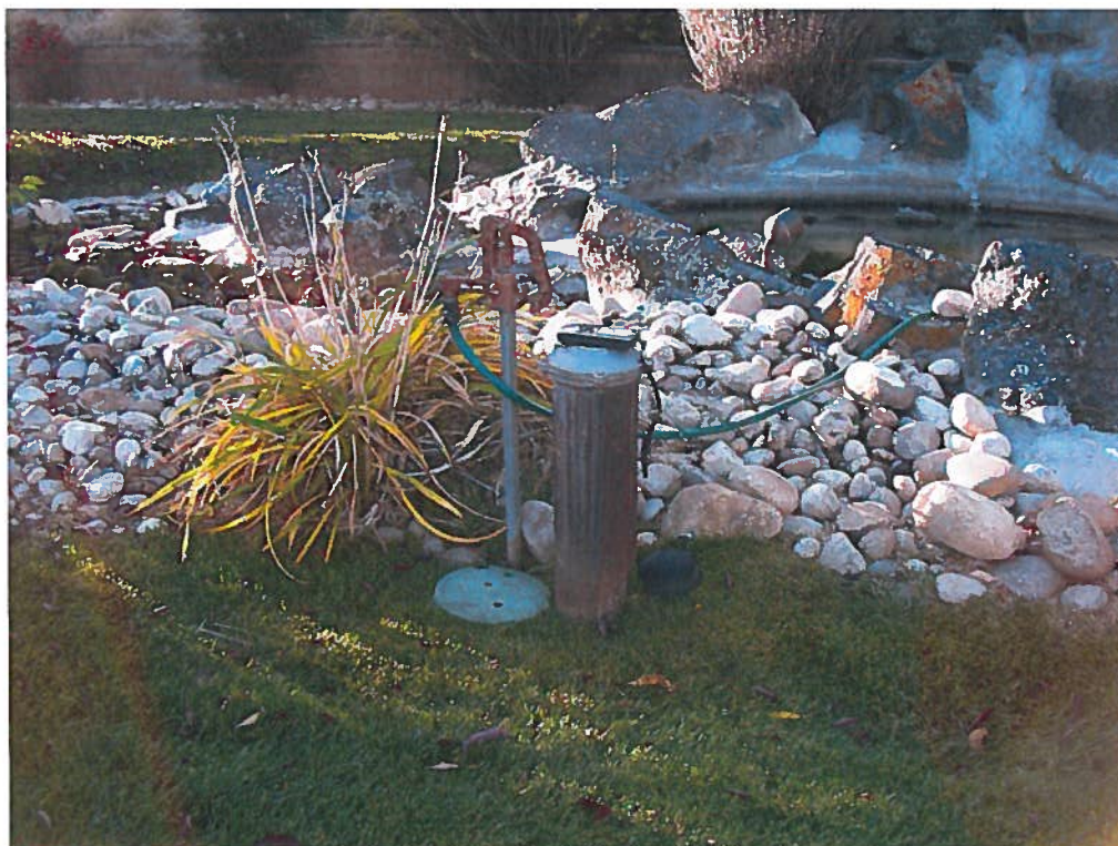
63-12592 Exam 11/2/2012: POD well in backyard facing south.
