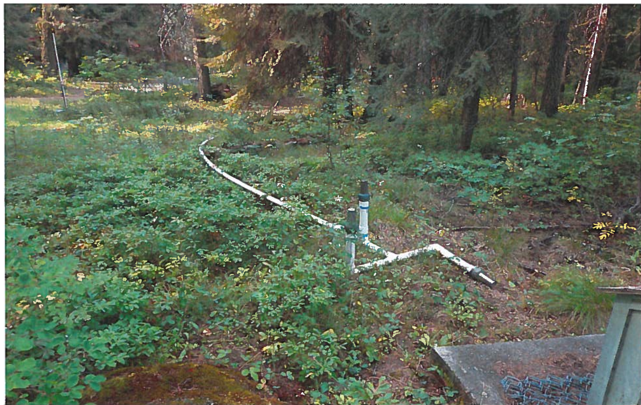
View of the 1 1/2" Polypipe 100' section of suction line. The right holder indicated that the irrigation system pumping from Payette Lake is used intermittently with the domestic system for irrigation of the property
