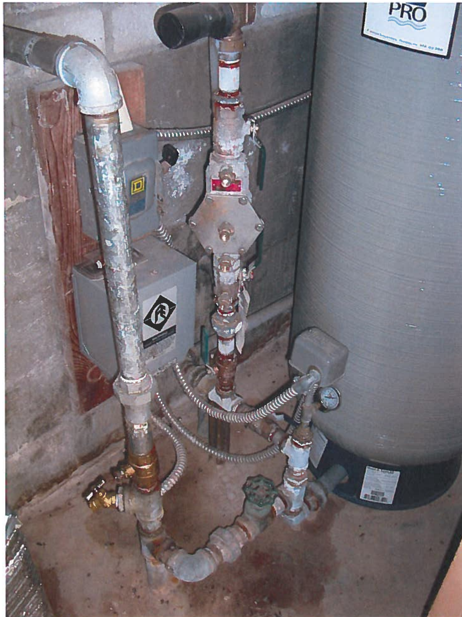
63-33272 Exam 8/27/2012: Diversion works inside pump house/shed. 2" line from production well on left side of photo. 1" line to heating system and domestic uses adjacent to pressure tank to right of 2" line from well.
