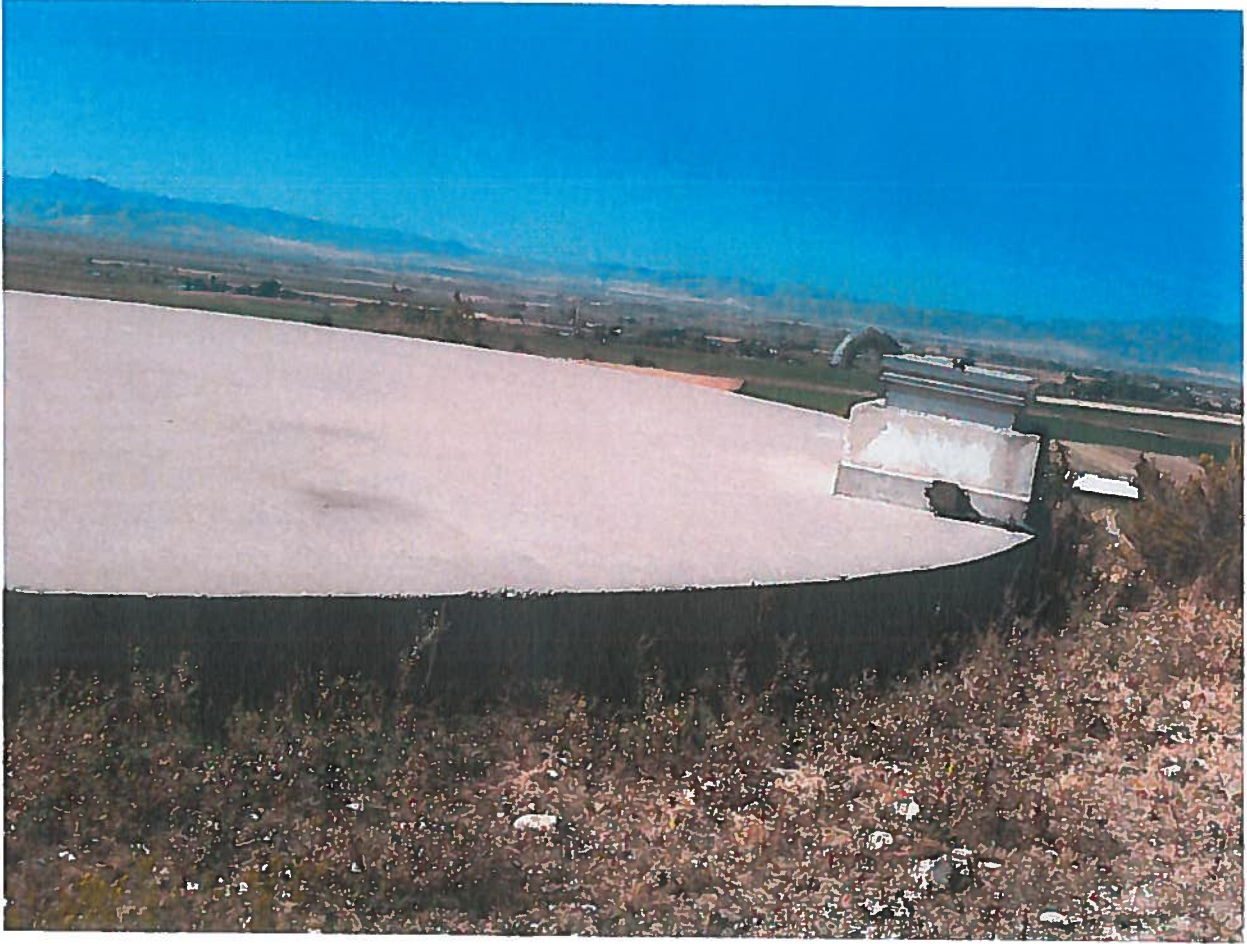
Storage tank above well #3
