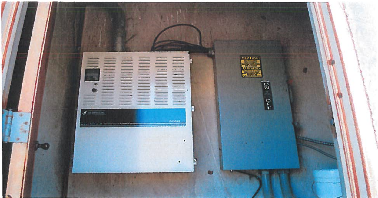
Pump house at Well above
