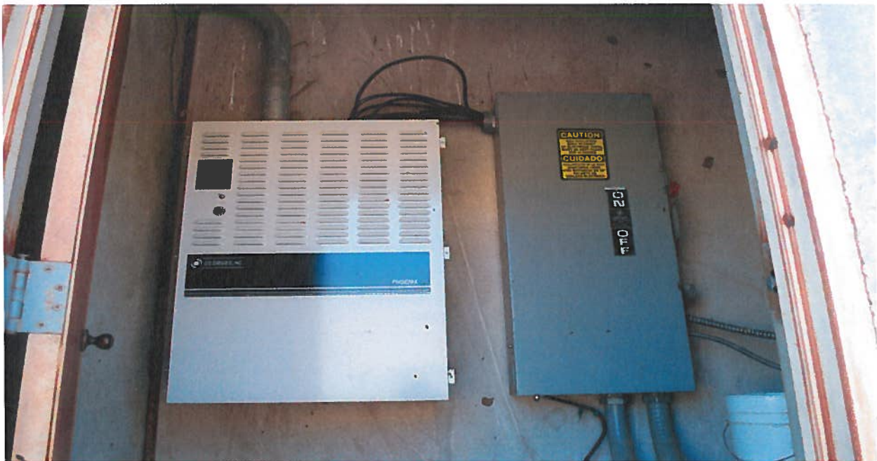
Pump house at Well above
