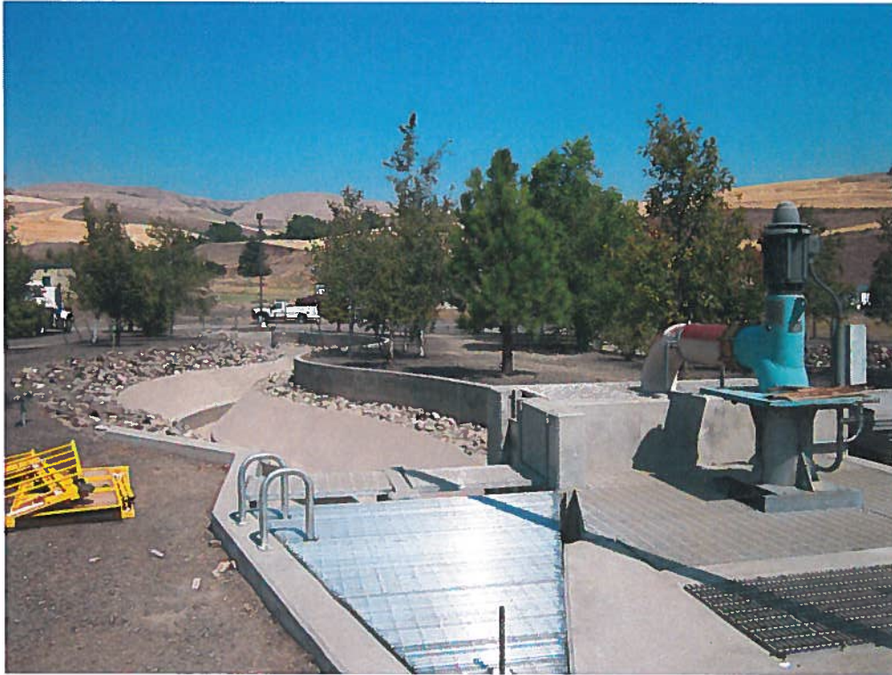
Photo #5. S-Curve raceways.
