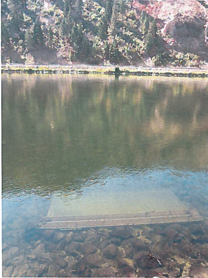
Photo #1. Photo of the surface water intake from the Clearwater River.
