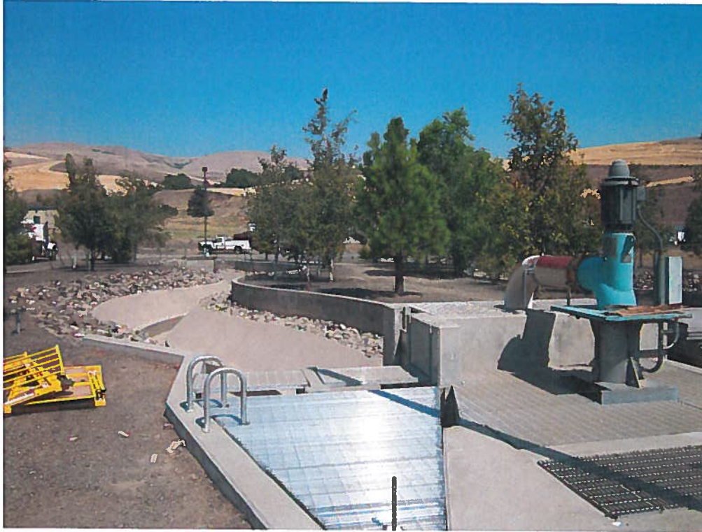
Photo #5. S-Curve raceways.
