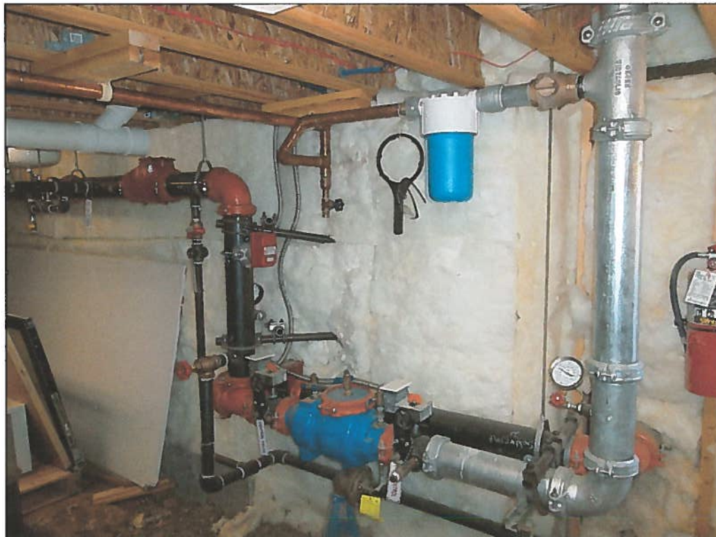
Crawl space of lodge – water line entry, filter and control devices
