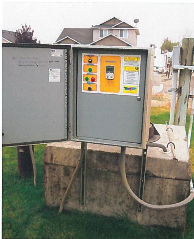
Licensed POD – Looking inside the power control box while the pump is running.
