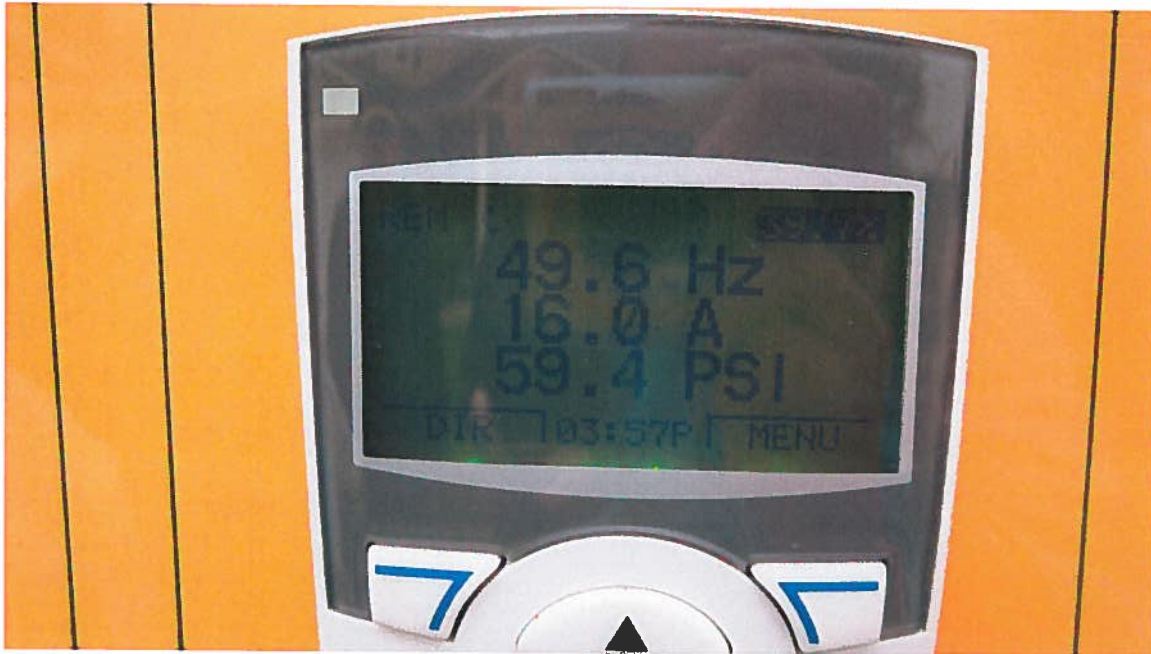
Close-up of the pressure gauge, 59.4 PSI during pumping.
