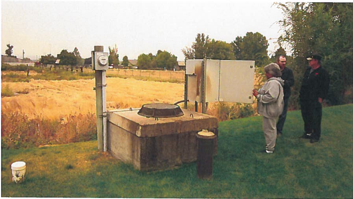
Licensed POD – Looking northwest at the concrete vault with pressurized tank, 8-inch well (#D0029613), and power control box. Water is pumped to sprinklers through buried pipes.
