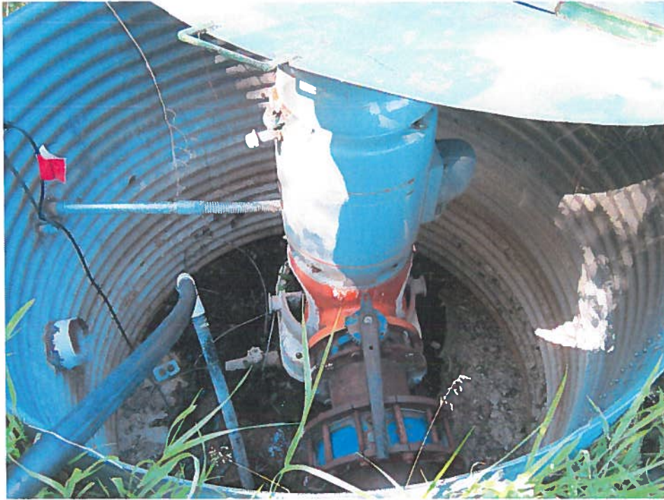
Figure 1: 40 Hp pump motor on well
