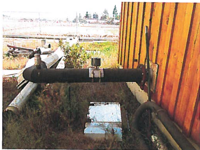
Photo 2. View of distribution system leaving the well house.
