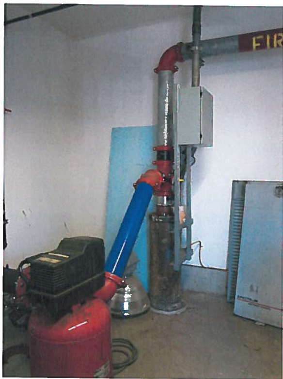
Photo 1. View of POD in the well house.
