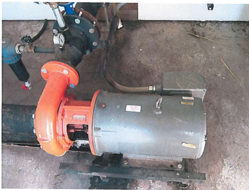
Photo 3. 30 Hp pump used to pump water for re-use.
