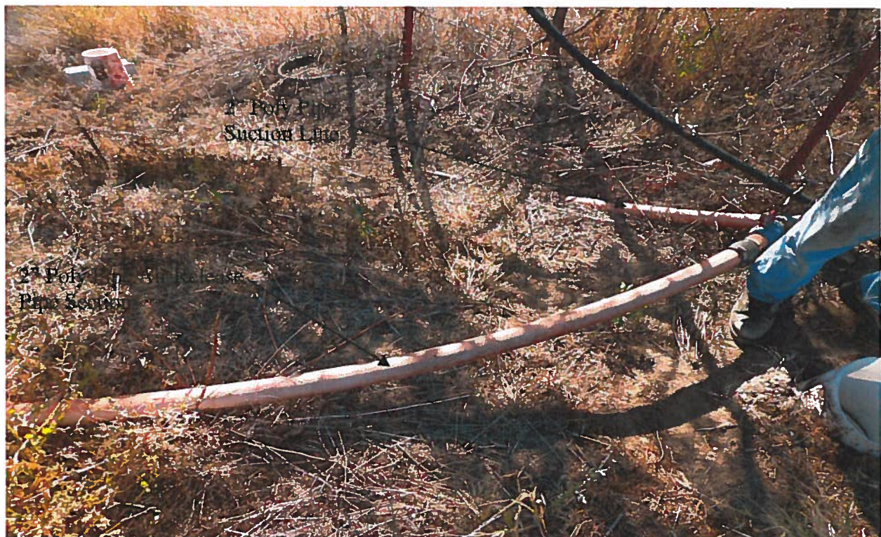
View of 2" poly pipe suction line to the 4,000 gallon water storage tank. The short section of 2" poly pipe with the control valve is used to release air when filling the water storage tanks. The buried 5-gallon bucket to the right contains a 1" isolation valve. The 1" line from the 4,000 gallon water storage tank provides water to the bathroom of the home for the operation of the toilets and showers.
