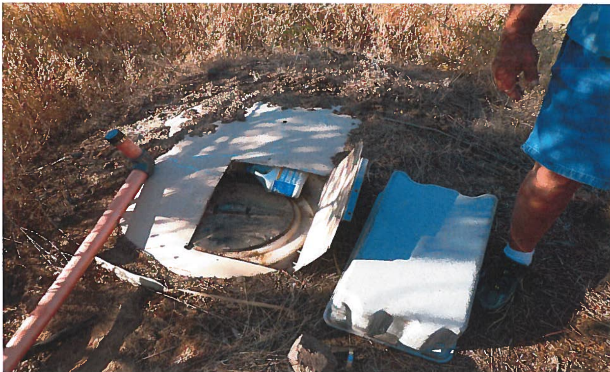
View of the buried 4,000 gallon water storage tank. The 4,000 gallon and 1,200 gallon water storage tanks are filled manually with the 2" suction line from the Salmon River.
