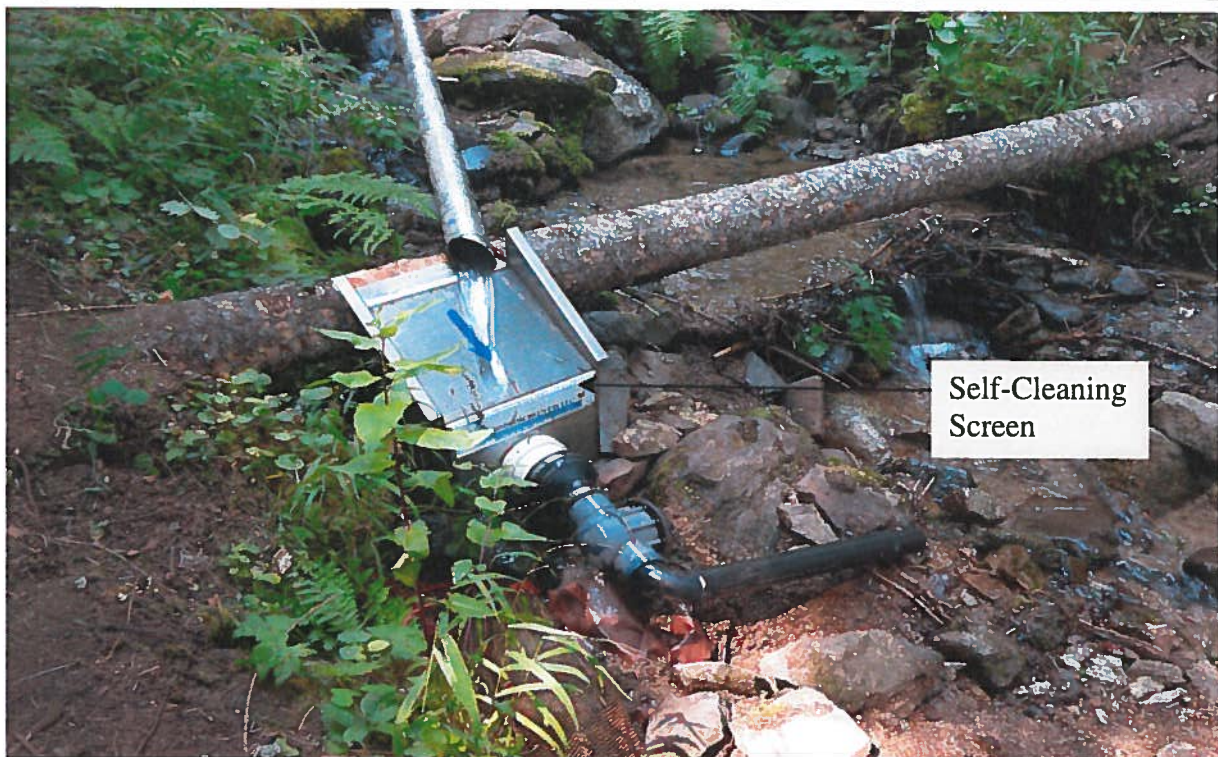
Point of Diversion: View of the 3" steel supply pipe discharging to a self cleaning screen. A short section of 2" PVC allows flushing and draining of the self-cleaning screen basin back to Alder Creek.
