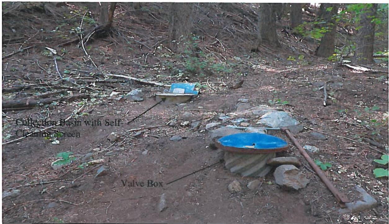
View of collection basin (in background) and valve box (CMP with blue lid). The collection basin contains another self-cleaning screen. The collection basin is located approximately 110 feet downstream of the dam. The control valve is used to periodically flush the debris from the collection basin and to drain the upper section of the pipeline back to Alder Creek.
