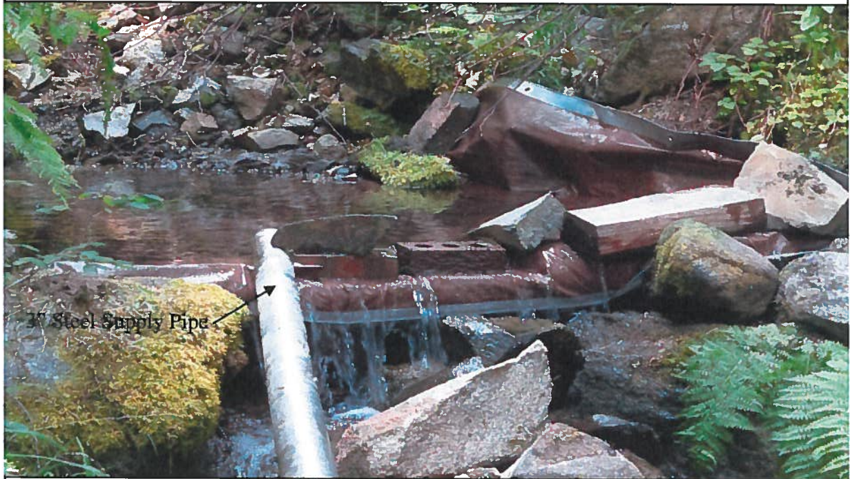
Point of Diversion: View of dam in Alder Creek and a 10-foot long section of 3" steel supply pipe. Water is discharged to a self-cleaning screen next to Alder Creek.
