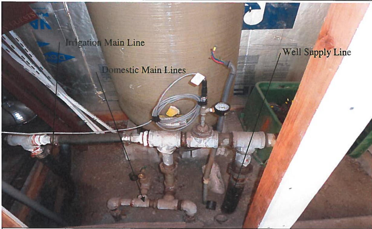
View inside of pump house of 1 1/2" PVC supply line from well, 1" domestic service lines, and 1 1/4" PVC irrigation main line. Operating pressure for the system is 62 psi.
