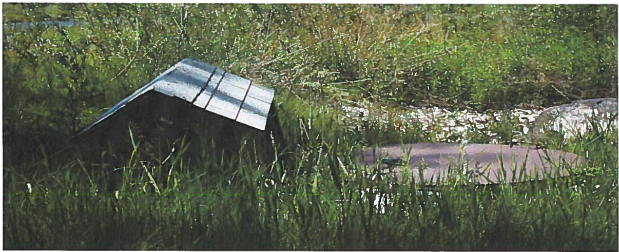
Pump and return flow tank
