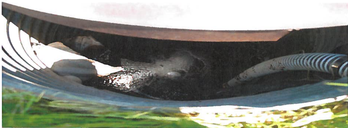
Return flow tank at Pond 2
