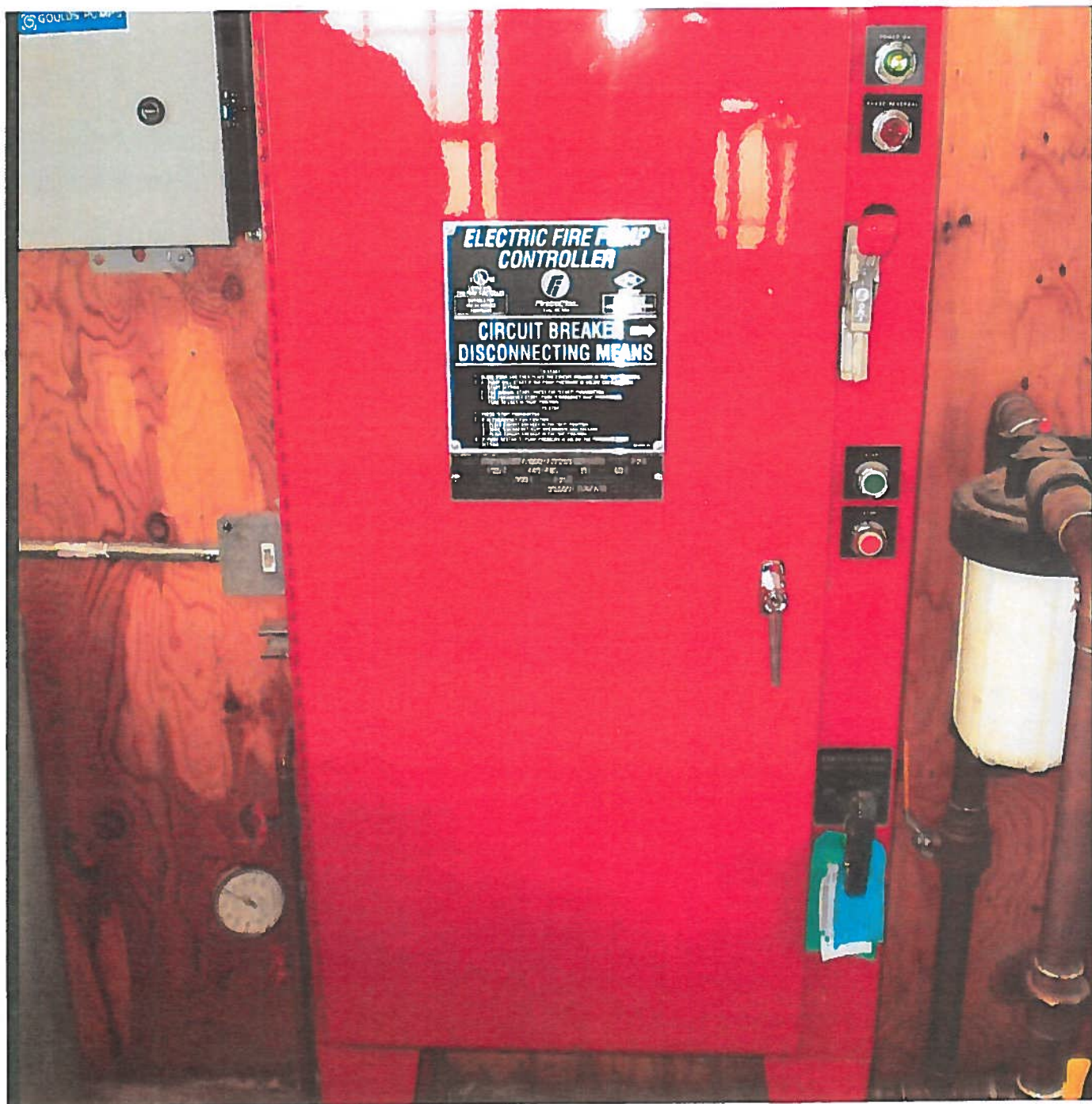
Fire system controls
