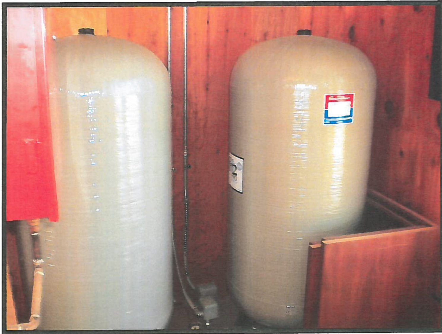
Domestic system pressure tanks
