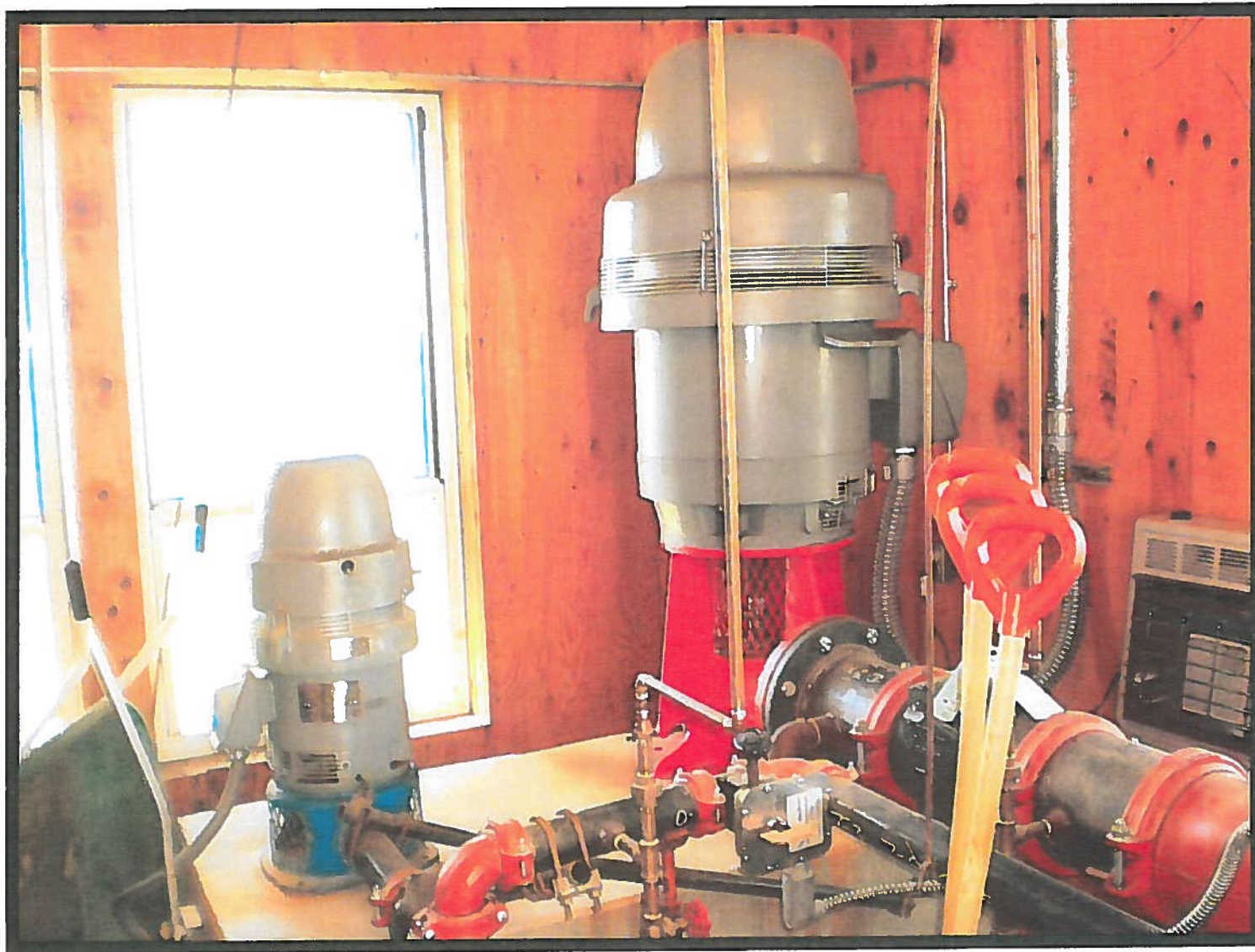
Fire system booster pumps
