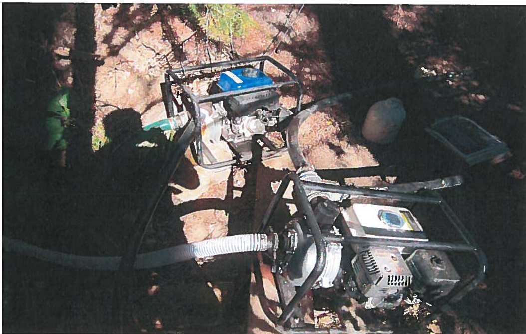
The 2 pumps on the bank of Fall Creek.
