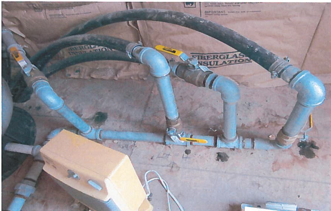
Photo of interior of pump house shows the black plastic pipe from the well [far left pipe] to the 1.25" steel pipe that goes to each of 3 pressure tanks, then back underground to the 3 black pipes that carries water to each of the homes.
