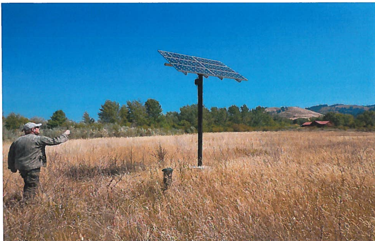
Point of Diversion: View northeasterly of backup well and solar energy system to operate the well pump.
